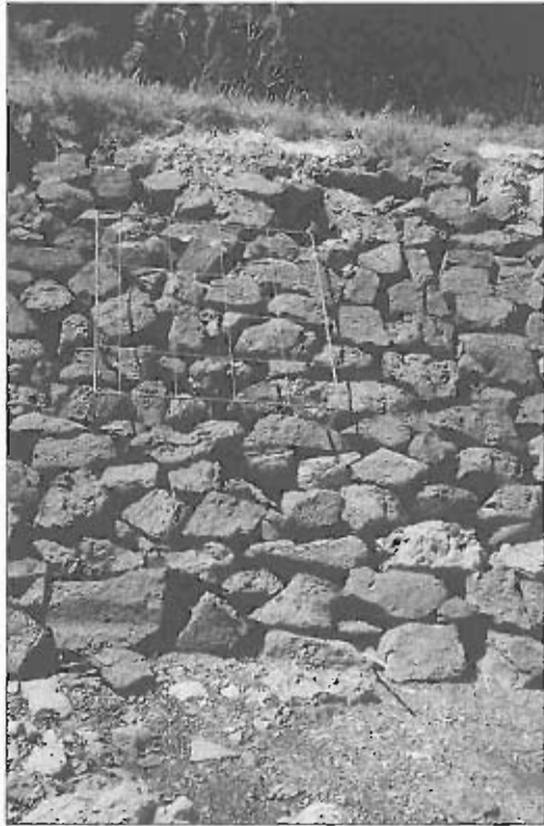
The Otago Harbour wall comprises over 37 km of hand-stacked stone walling, holding up the roads and the railway along the harbour edge. This representative section shows that the stones were laid to an even face, but they were not graded in size from top to bottom.
