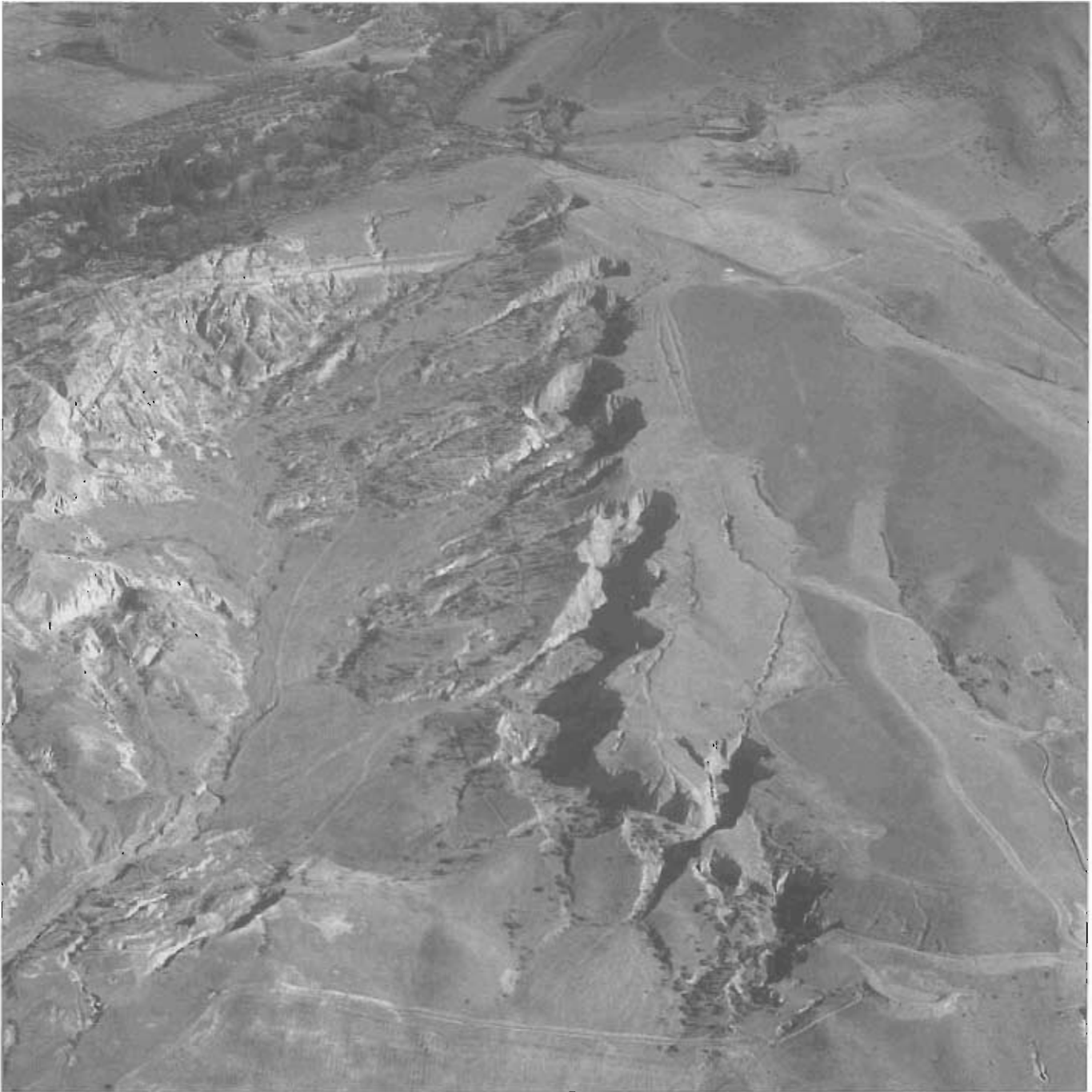
from them to each party's hydraulic sluicing nozzle. The sludge channel in Pipeelay Gully runs up from the road to the left of the photograph and right across the background.
