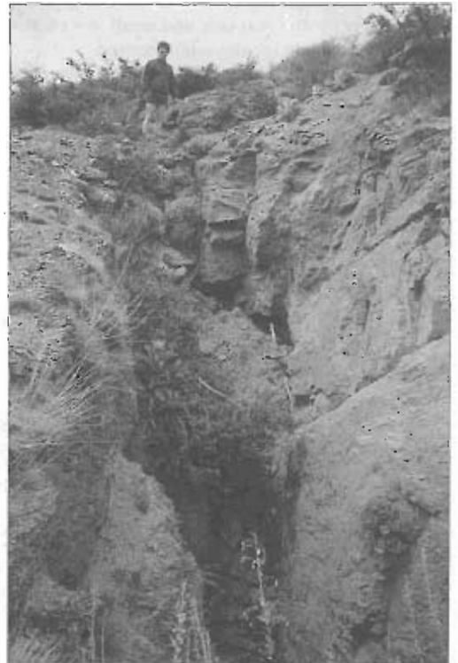
A massive collapsed adit of the Caledonian Mine, running under the Carricktown Road (right). The mullock heap from it lies high-right in the photograph of Battery Creek, on the left. Photograph: DOC files, Dunedin
