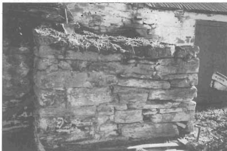
A bread oven built into the chimney wall of the men's quarters at Lauder.
