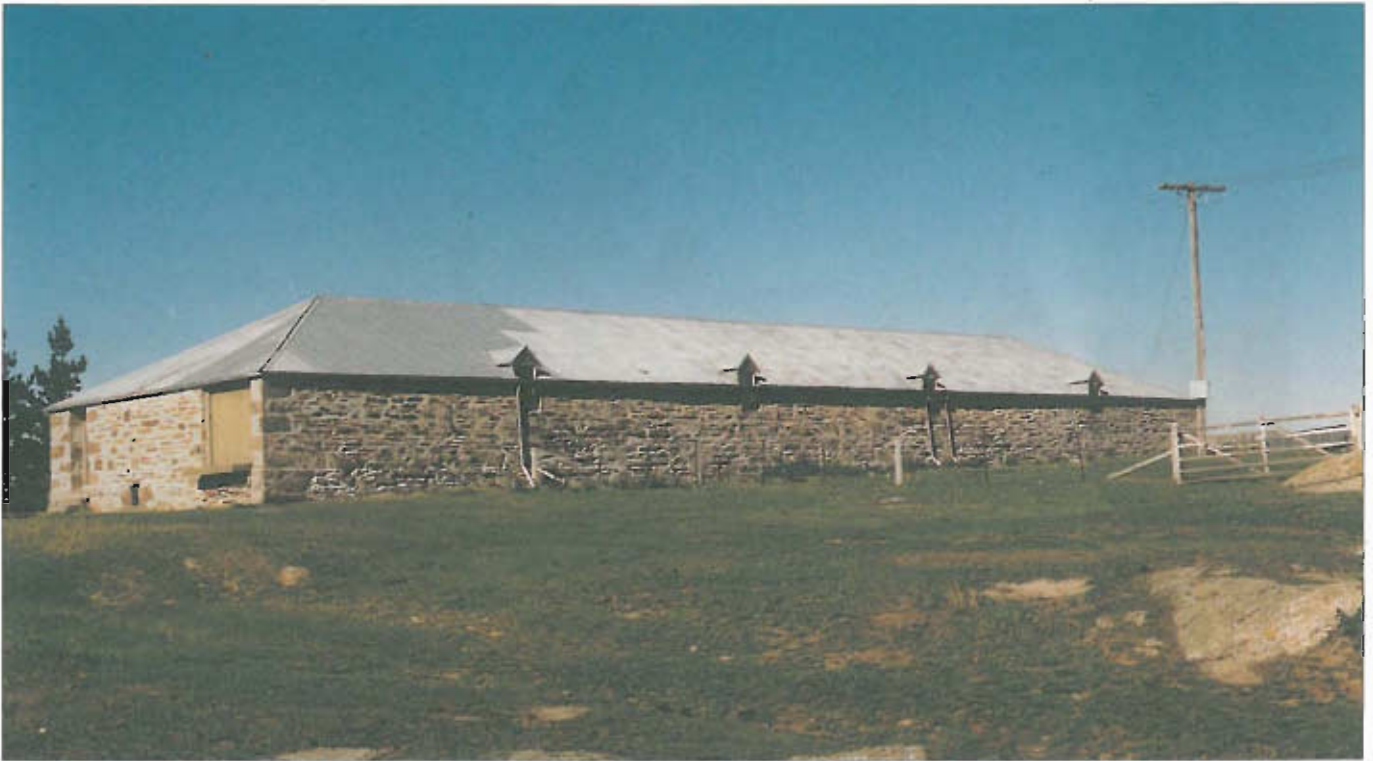
The stone woolshed of Cottesbrook, near Middlemarch, was built about 1867 from schist slabs. It accommodated only 24 blade shearers, a small number for such a large property.
