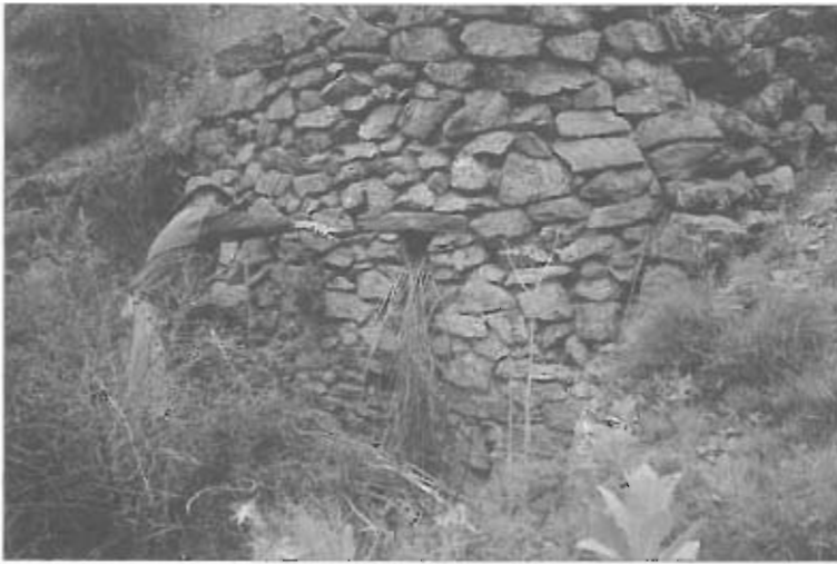
Large stone dams with carefully constructed outlets were built in Battery Creek as part of the water-control systems for the Carricktown batteries.
