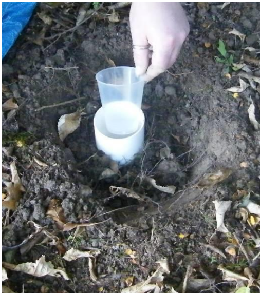
Figure 5. Place a cup in the downpipe to collect overflow soil before building up and packing down the soil up to the lip of the downpipe.
