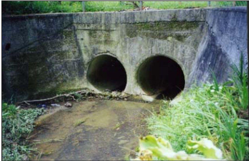
Plate 3. Vertical headwall. The rounding of the headwall so that it gradually meets the banks reduces entrance velocity changes and improves fish passage.
