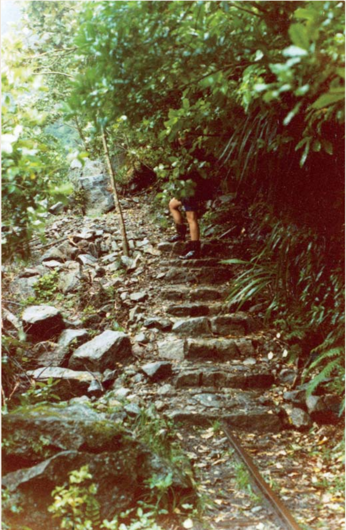
Photo 26: Rock slip over tramway (between 'bridges 3 and 4'. Walkway follows stone steps over slip ca 1978
