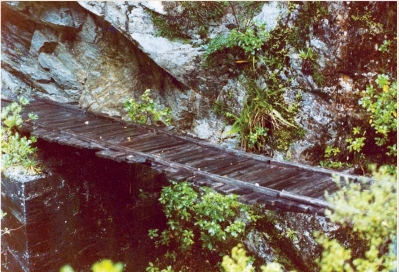
Photo 25: Bridge west of tunnel (probably Irishman's Tunnel), showing lack of stringers and concrete foundations in ca 1978.
