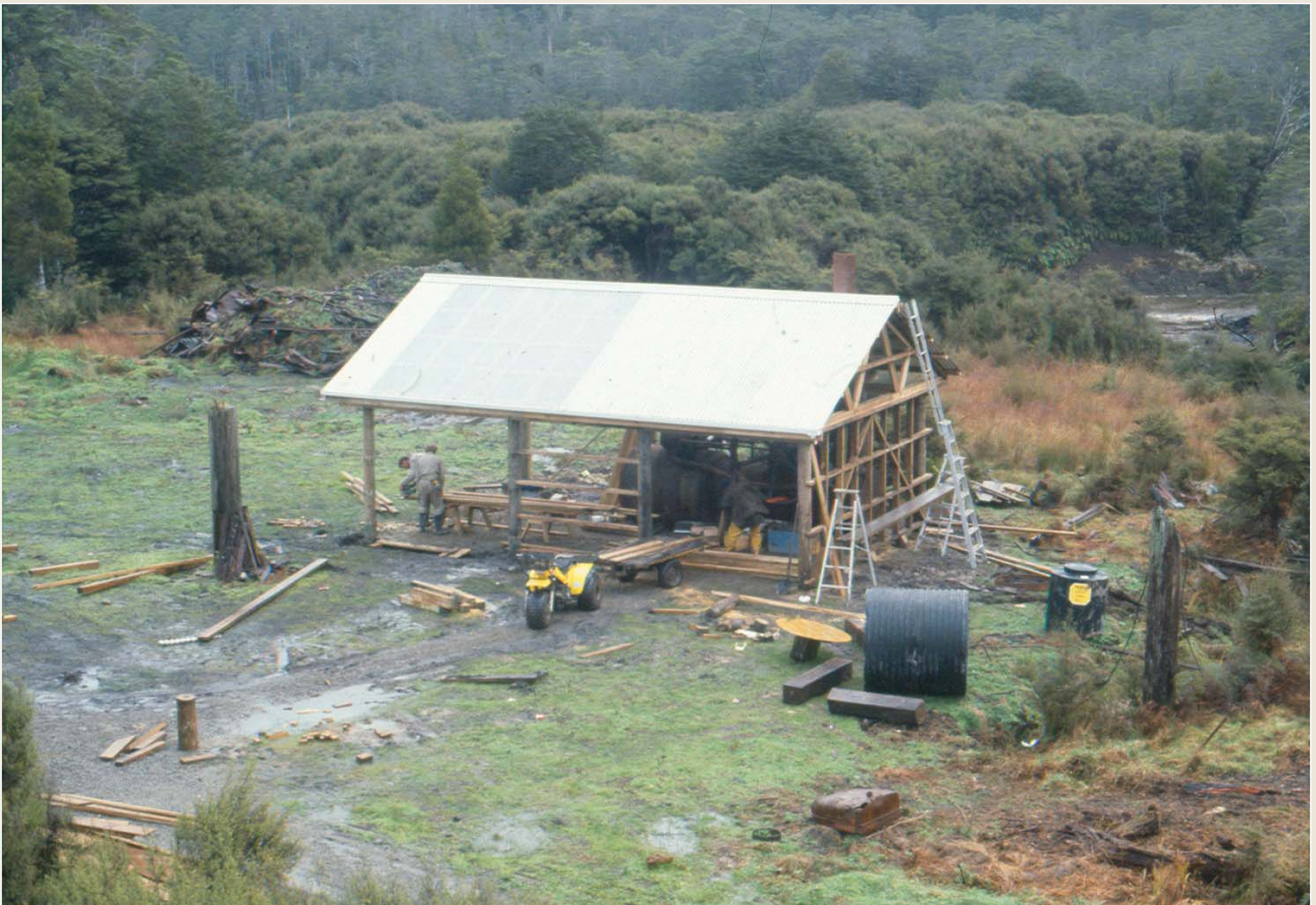
Photos 31 and 32: Before and after shots of the Mumm's Mill site during the construction of the shelter over the mille steam engine.
