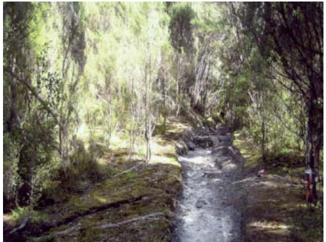
Figure 9: Condition of the modified section at the start of the track - run off to coal prospecting site to the left of the image.
