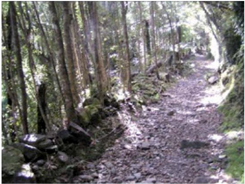
Figure 30: Rock retaining wall 1. Section one of the track showing sapling growth along the outer edge.
