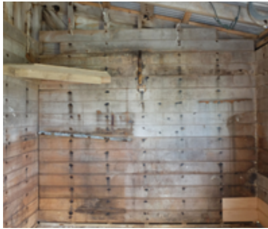
Figure 59. The inside north wall of the castaway depot hut, 2018. The line where the Président Félix Faure castaways' bunks were built is clearly visible half-way up the wall. Photo: Peter Petchey.
