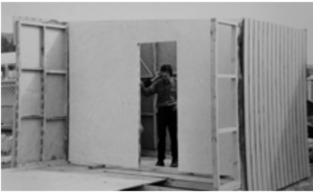
Figure 17. Trial construction of the 1978 BAAS hut at Tūrangi, prior to it being broken down for transport. Photo: Newton 1979; Archives New Zealand Te Rua Mahara o te Kawanatanga, Dunedin Regional Office.
