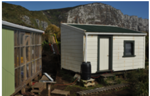
Figure 51. The castaway depot hut adjacent to the 1978 BAAS hut after the repair works on the latter were completed in 2015. The castaway hut is in good condition, but the staining from rusting nails is evident. Photo: Kath Walker.
