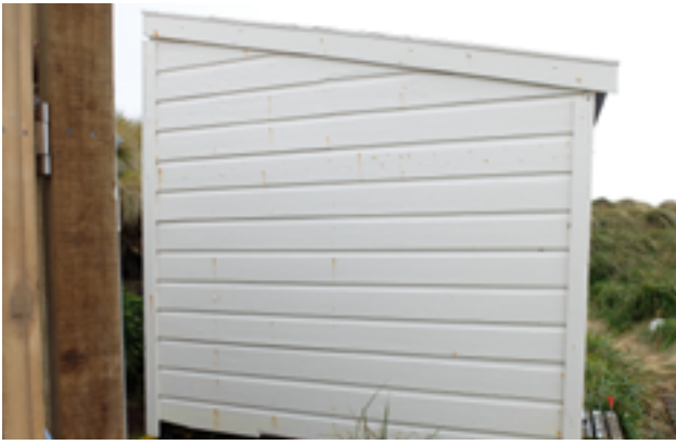
Figure 55. South wall of the castaway depot hut, 2018, showing the nails in the fifth weatherboard from the top that fixed the lean-to roof constructed by the Président Félix Faure castaways. Photo: Peter Petchey.
