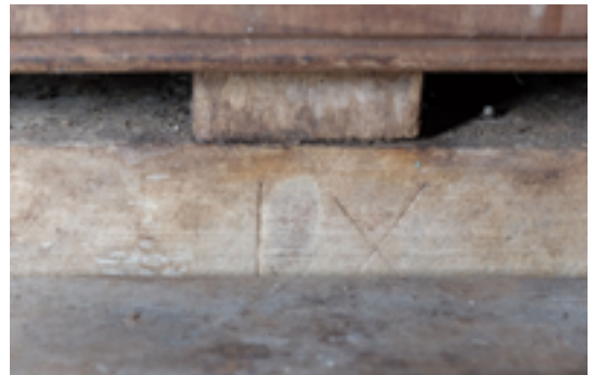
Figure 69. Bottom plate and base of stud in the west (rear) wall of the castaway depot hut, 2018, showing one of the Roman numerals that the timbers were marked with to aid reassembly of the prefabricated structure. Photo: Peter Petchev.
