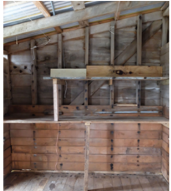
Figure 60. The inside south wall interior of the castaway depot hut in 2018 showing the modern shelving which is constructed partly of wall lining boards taken from the wall. The wall framing, including the brace, is also clearly visible in this view. Photo: Peter Petchey.
