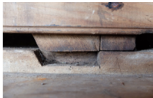
Figure 73. Bottom plate of the west (rear) wall of the depot, 2018, showing the rebate cut for the bottom end of one of the wall braces. The brace has pulled out of the rebate, suggesting that the building has moved slightly over time. Photo: Peter Petchey.
