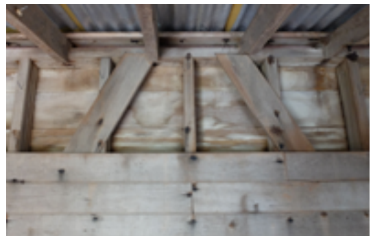
Figure 71. Top middle of the west (rear) wall of the castaway depot hut, showing the studs, top plate and bracing in the wall, with the rafters attached to the top plate, 2018. Photo: Peter Petchev.
