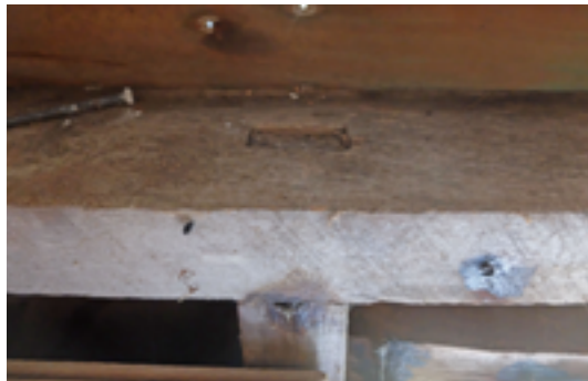
Figure 68. Top plate and stud in the east (front) wall of the castaway depot hut, showing the mortise and tenon joint, 2018. Photo: Peter Petchev.
