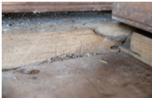
Figure 70. Scarf joint in the bottom plate of the west (rear) and north side wall of the castaway depot hut, 2018, with Roman numerals to aid reassembly. Photo: Peter Petchev.
