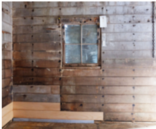
Figure 61. The inside east (front) wall of the castaway depot hut in 2018 showing the hut's one window (north side of the door). Replacement tongue and groove lining boards are visible in the lower left (northeast) corner. Photo: Peter Petchey.
