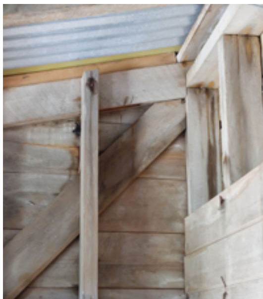
Figure 72. Top left hand (southwest) corner of the castaway depot hut, 2018, showing the side wall studs and bracing. Note the lack of a top plate on the side wall, with the studs fixed to the end rafter instead. Photo: Peter Petchey.
