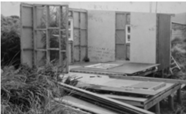
Figure 19. The new BAAS hut during construction on Antipodes Island in 1978. Photo: Newton 1979; Archives New Zealand Te Rua Mahara o te Kawanatanga, Dunedin Regional Office.
