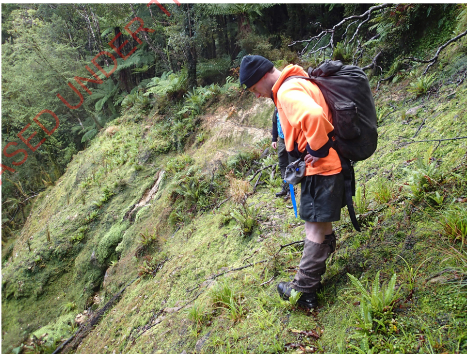
Figure 17. An area where the original line of the track has been destroyed by slips.
