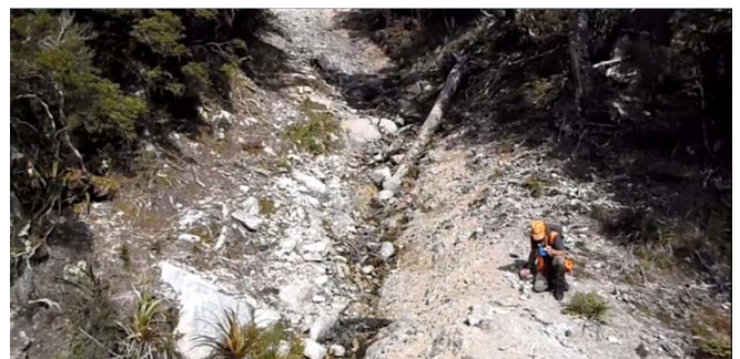
Figure 12: One of the many small "guts" that are a feature of the section of track on the top of Pike Ridge. From a construction perspective these are easily managed via small boardwalks or stacked stone seep culverts as needed.
