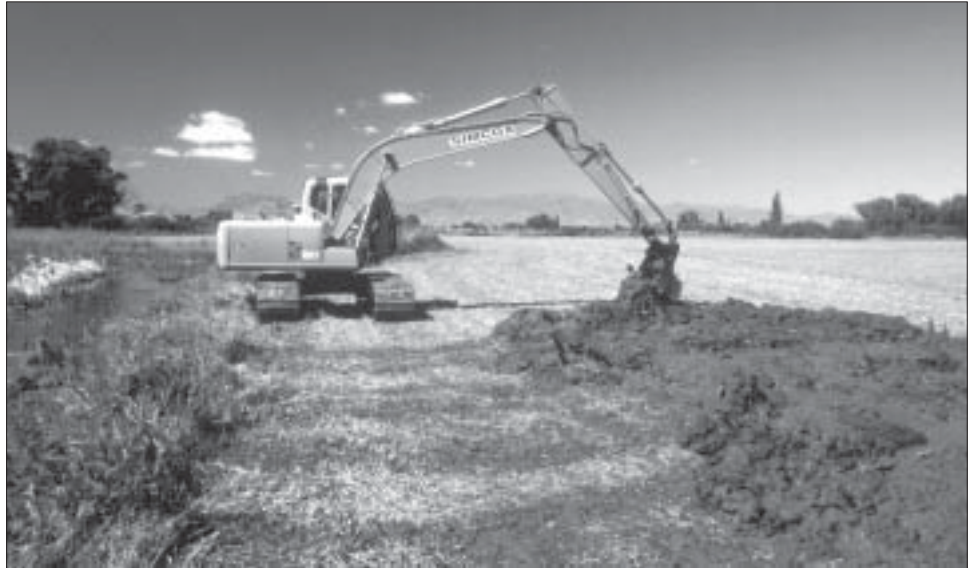
Figure 3. Excavated weed and sediment should be placed close to the bank to enable eels and crayfish to return to the drain.
