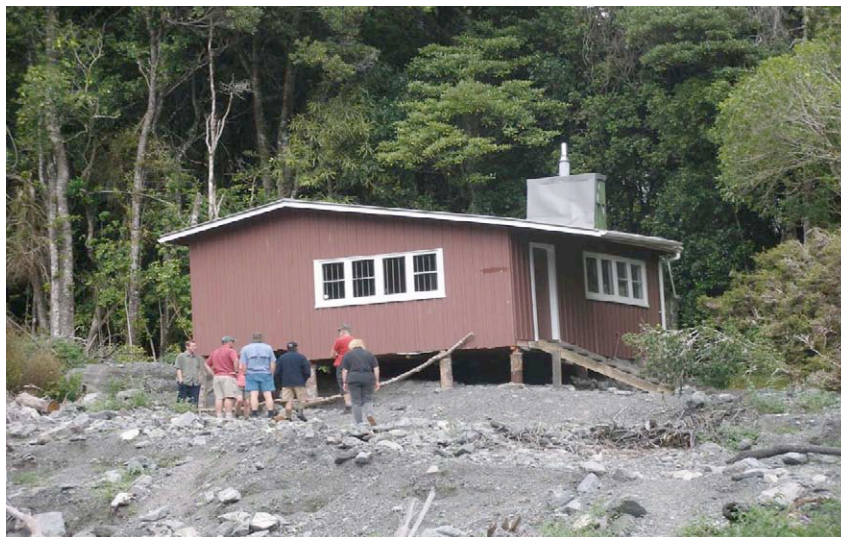
Wellington Conservation Board members inspecting the storm damaged Tararua Tramping Club hut in the Orongorongo Valley
