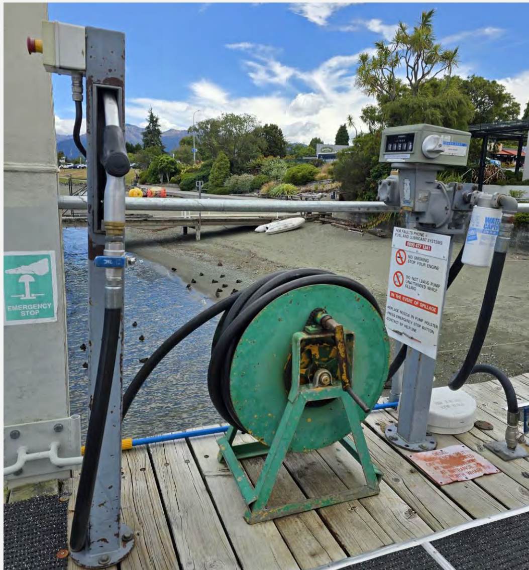
Figure 16 – photo of fuel installation
