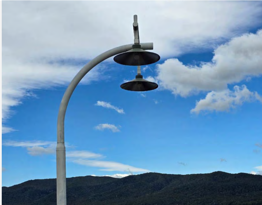
Figure 15 – photo of jetty lighting
