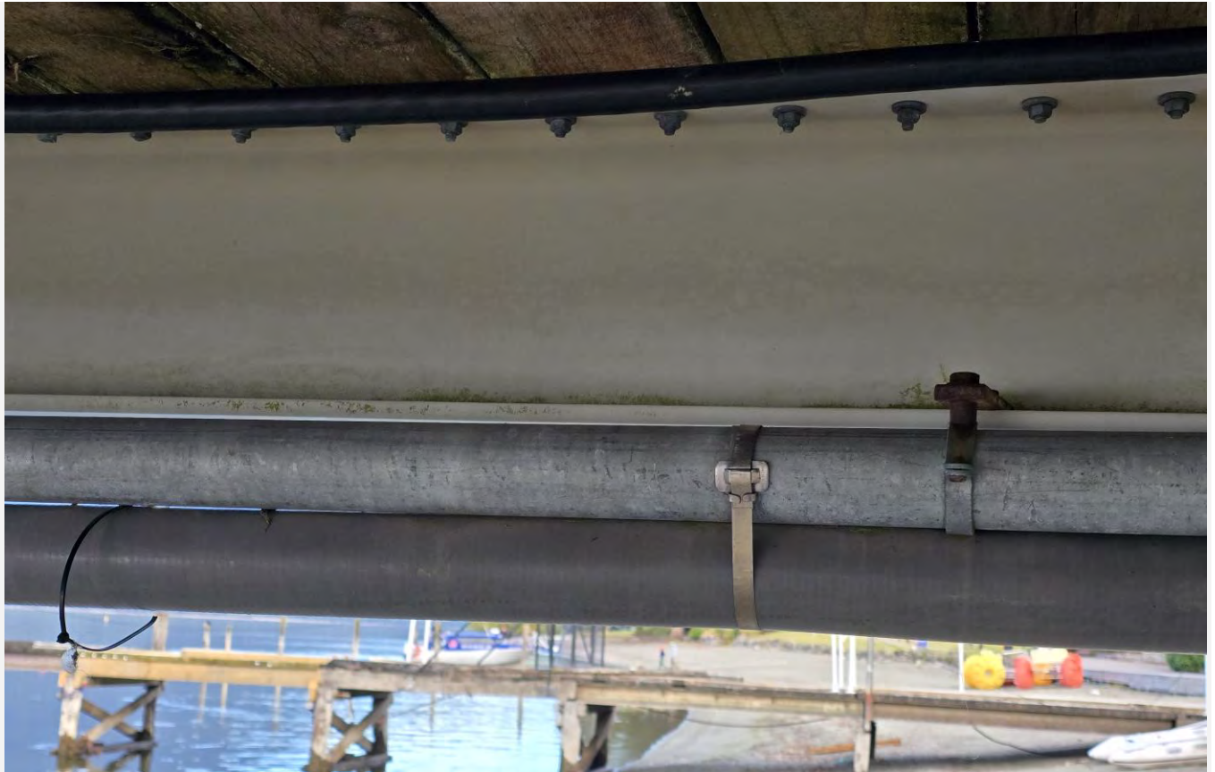
Figure 21 – photo of the services under the jetty – water, sullage and fuel
