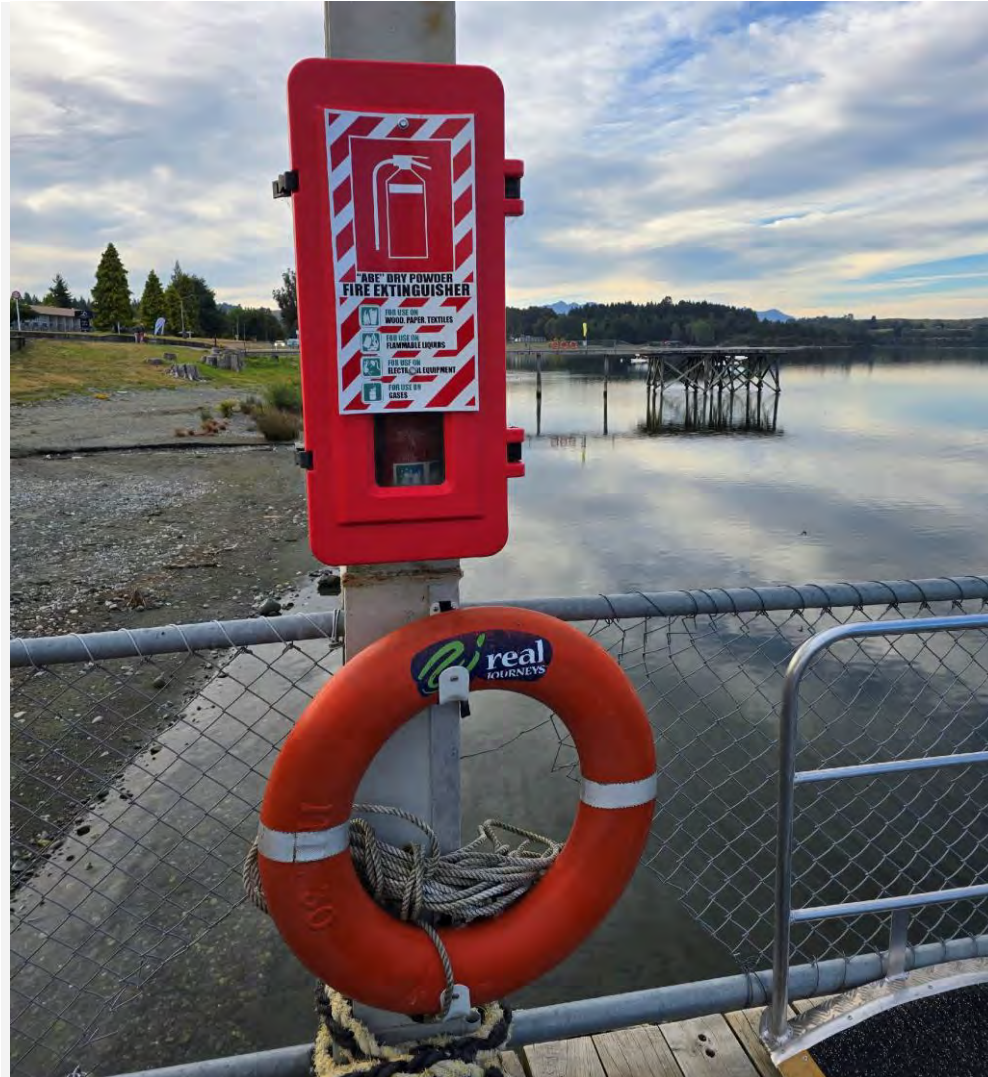
Figure 19 – photo of fire extinguisher and life ring
