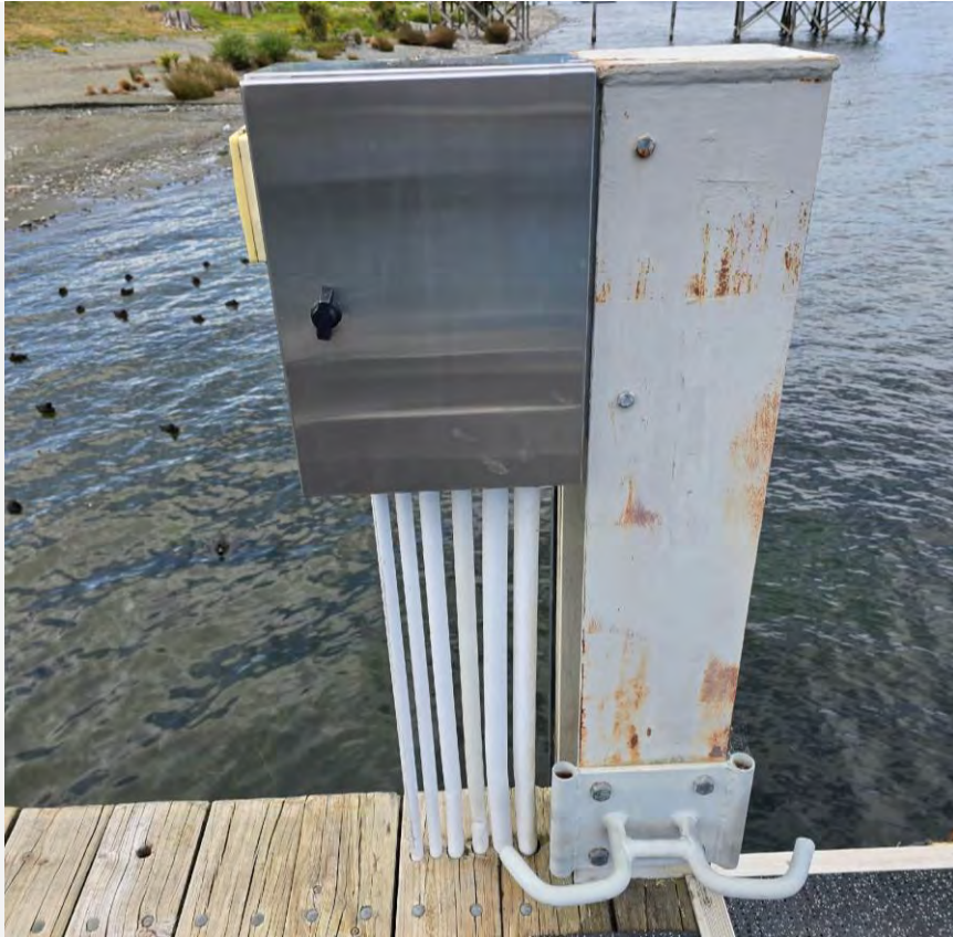
Figure 23 – photo of jetty electrical panel
