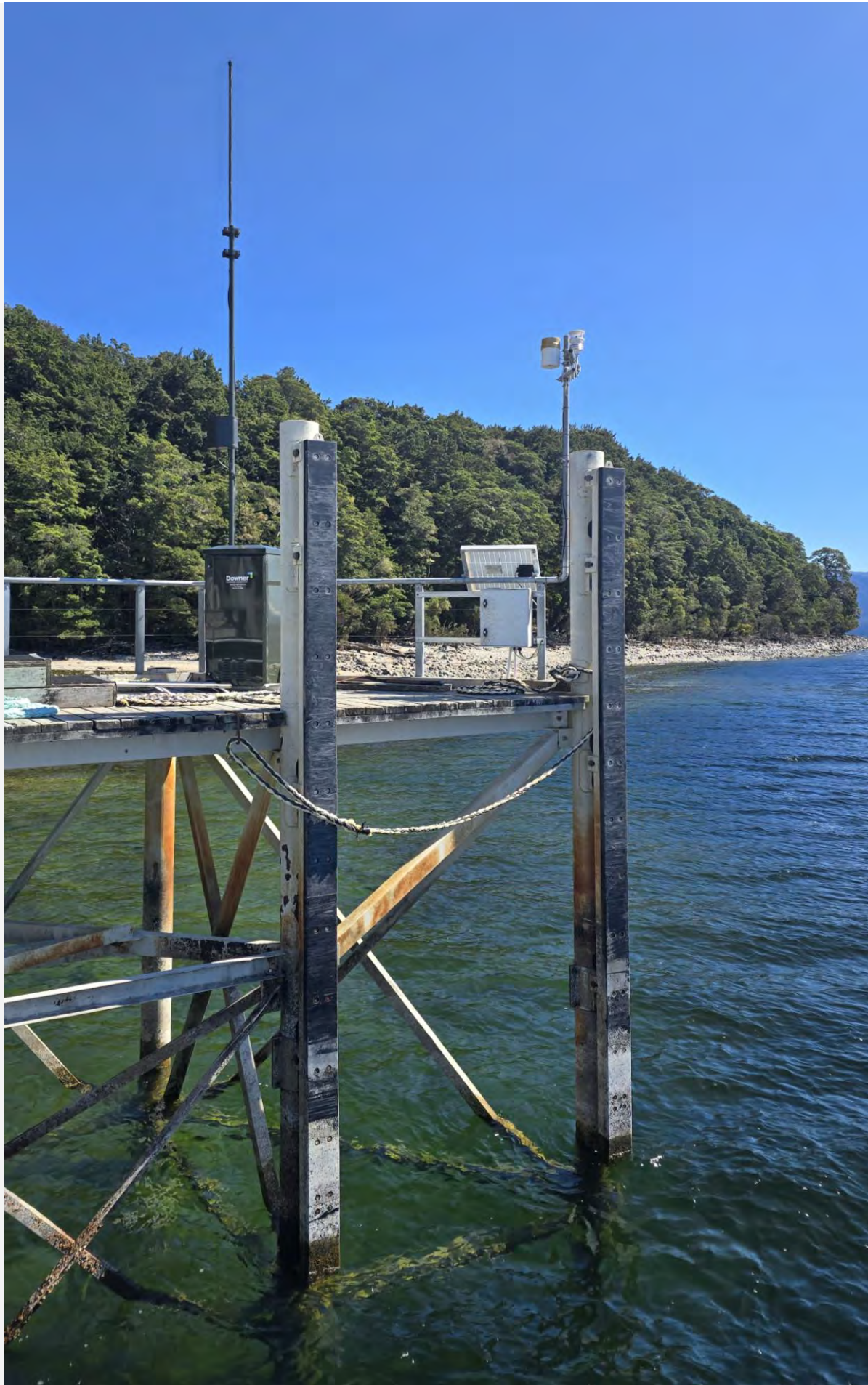
Figure 34 – photo of the 2x telecommunications equipment on the Te Ana-au Glowworm Caves wharf
