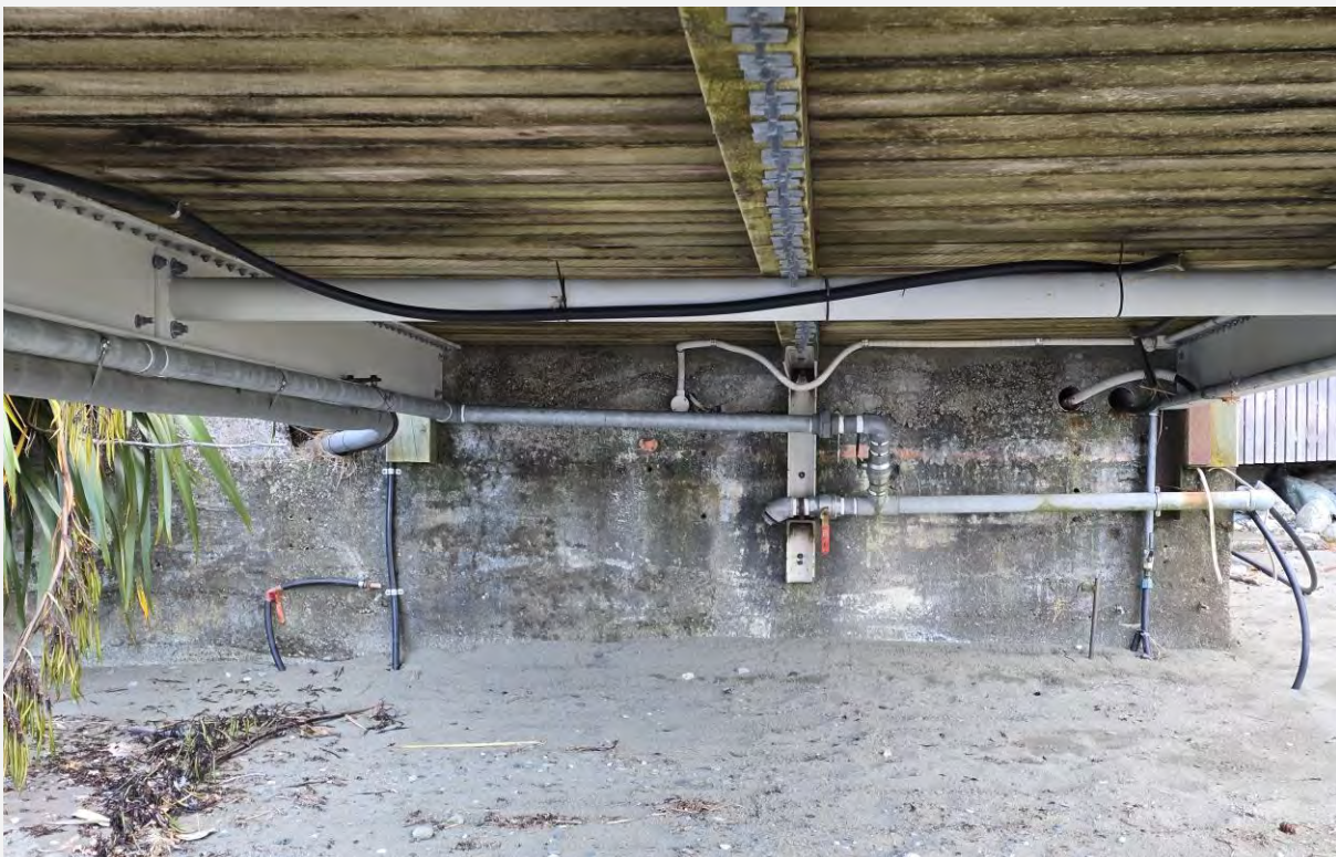
Figure 20 – photo of the services under the jetty – fuel, sullage, water and electricity
