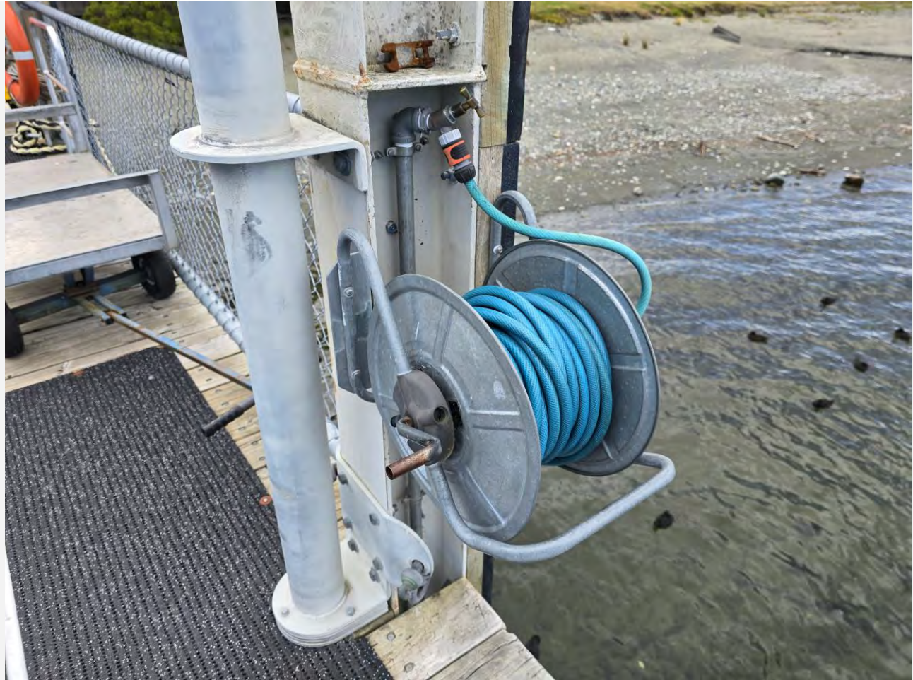
Figure 25 – photo of freshwater supply
