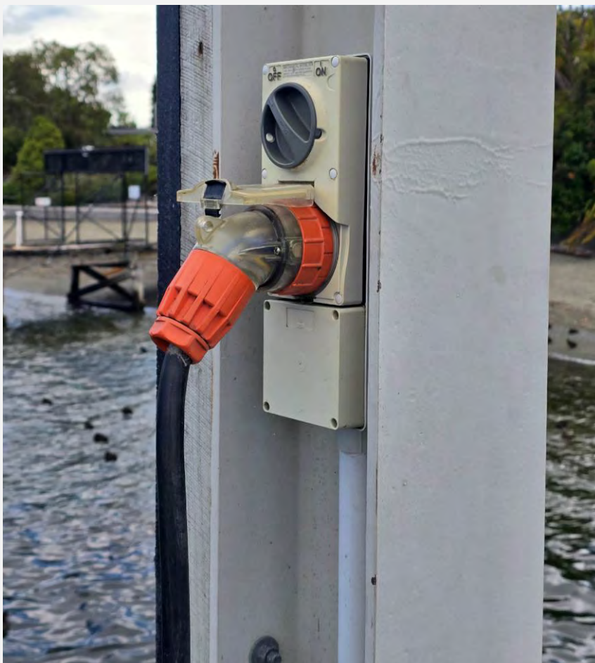
Figure 22 – photo of vessel shore power cable connection
