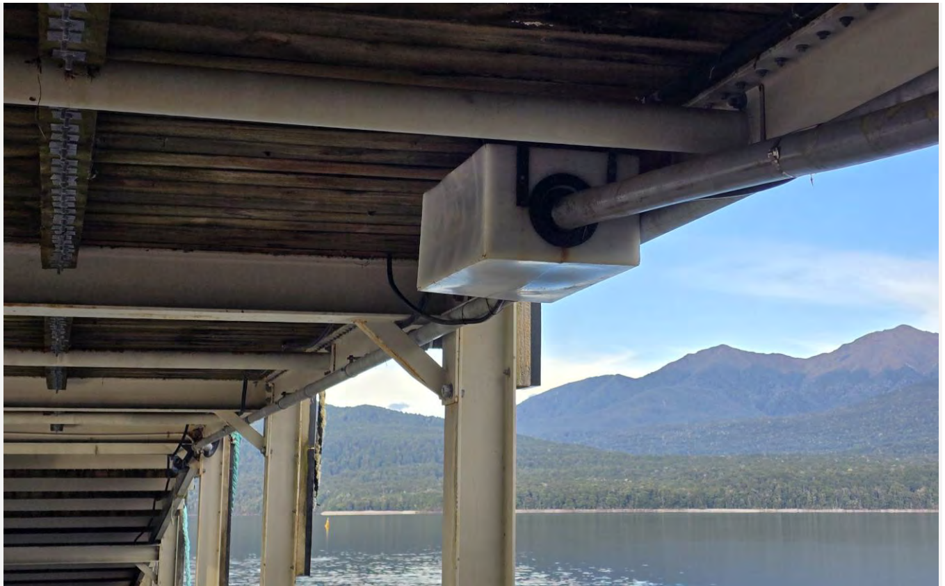
Figure 17 – photo of the fuel installation under the jetty
