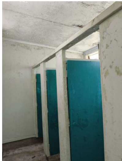
Figure 2-2f: Some ancillary buildings require repair or replacement
