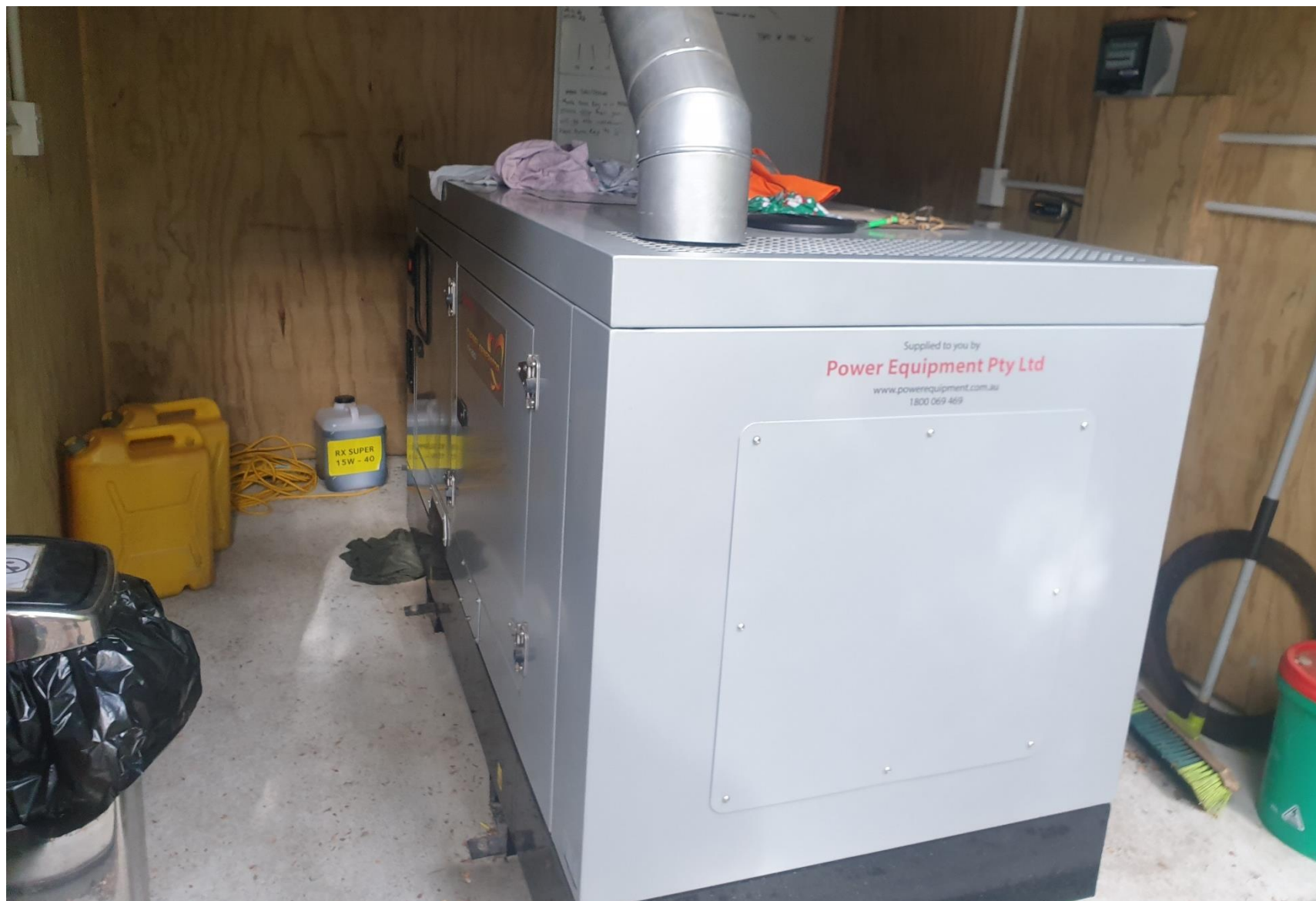
Figure 44. Photo of Yanmar generator
