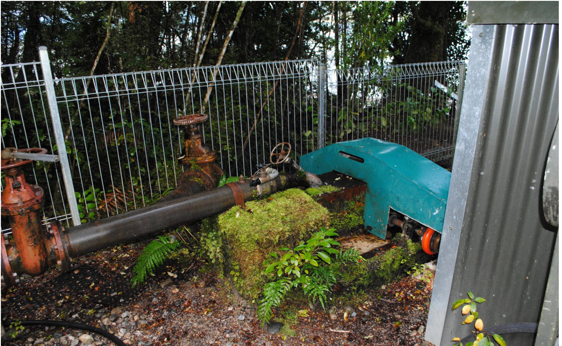
Figure 38. Photo of Hydro inside enclosure
