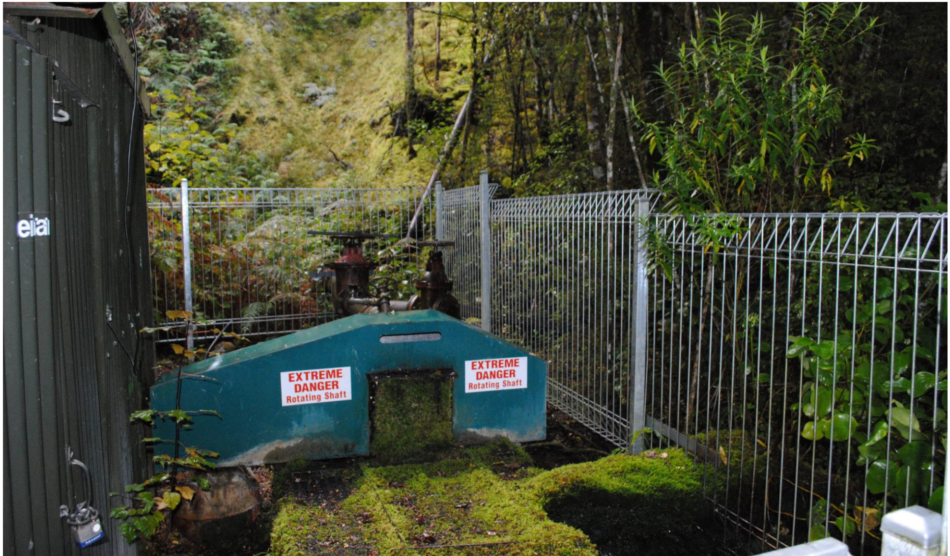
Figure 37. Hydro including its enclosure
