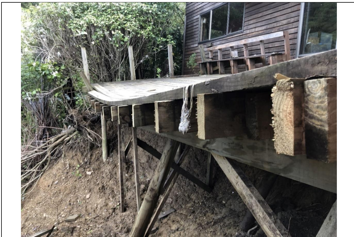
Photograph 2: Damaged timber deck (front portion removed following landslip) and back scarp of landslip.
