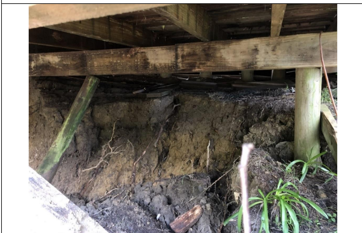
Photograph 3: Underside of timber deck and back scarp of landslip.
