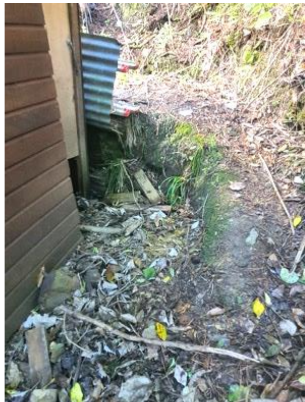
Figure 6: View of the minor unretained cut face to the rear of the dwelling.
