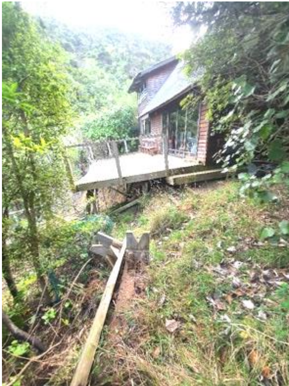
Figure 3: View of the dwelling and remaining damaged deck, looking north from site access track.
