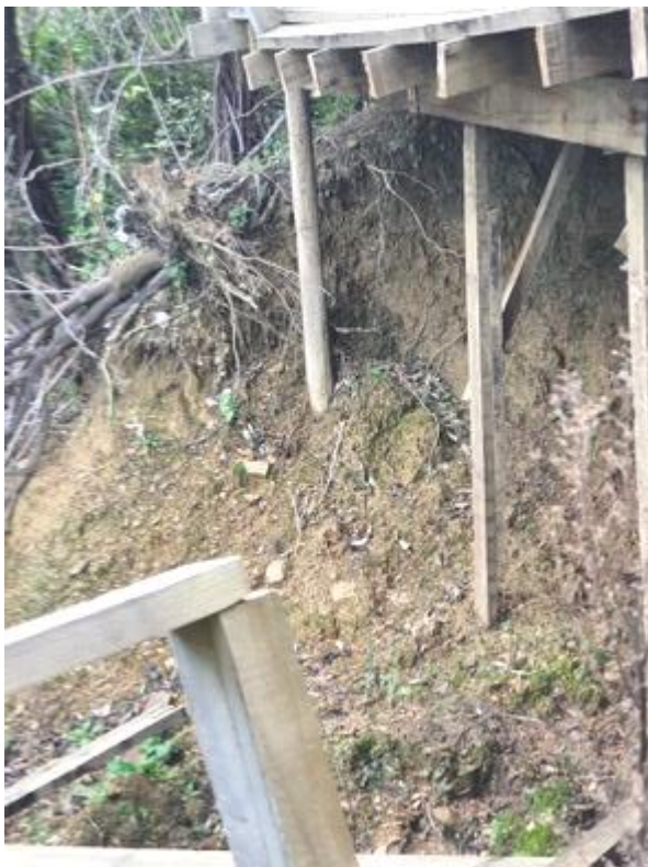
Figure 5: View of the head scarp, showing predominantly silt material with minor schist cobbles.
