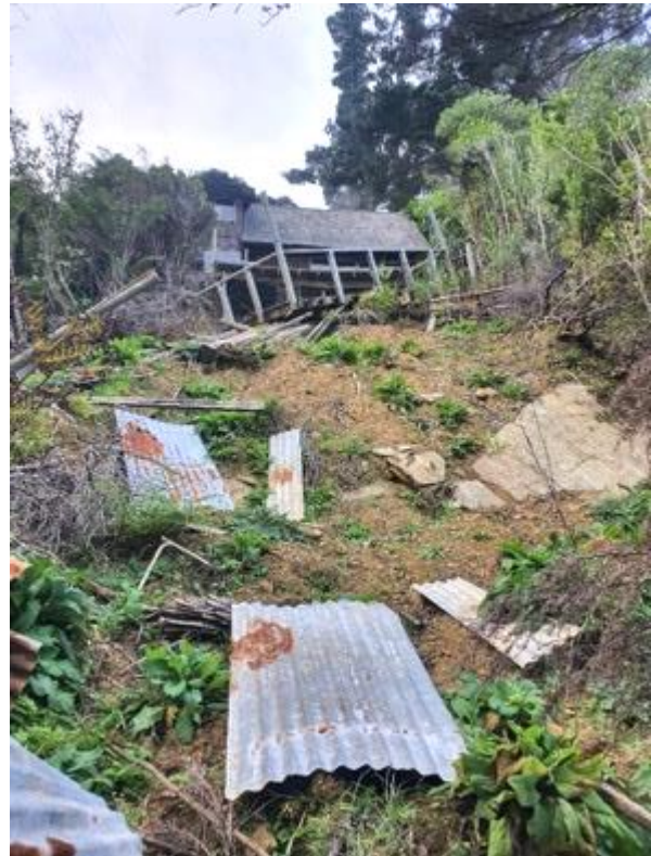
Figure 4: View of landslide debris from the shoreline (exposed schist bedrock on right).
