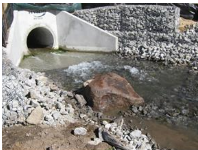
Figure1. New replacement culvert installed in Waiowhero Stream, Rotorua, early in remediation process showing shallow, high velocity water spilling from concrete apron.
