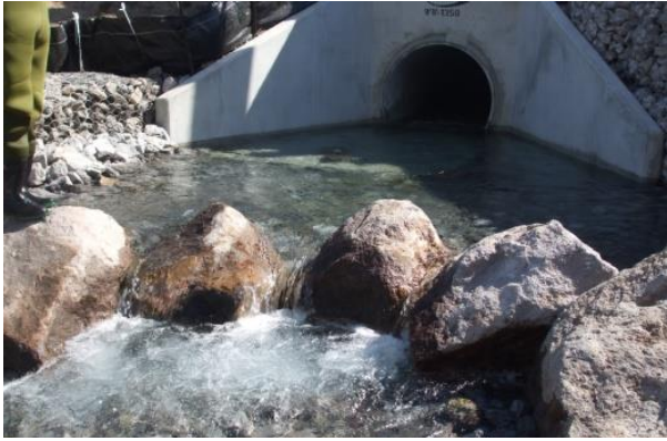
Figure 2. New replacement culvert installed in Waiowhero Stream, Rotorua, with the upstream facing 'V' weir downstream (March 2010. Photo: John Meikle)
