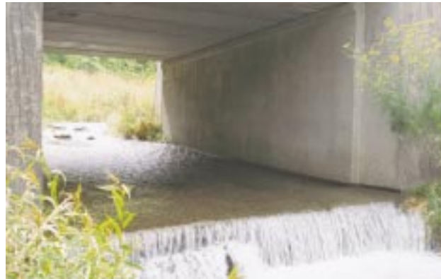
The overhang and level positioning of this concrete bridge apron will prevent most fish from swimming upstream.
