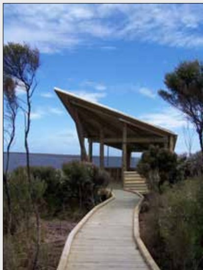
Waituna walking trail under construction, and the viewing shelter that connects with the new track.
