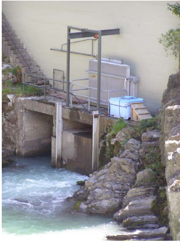
Waihopai Power station trap (blue box).
