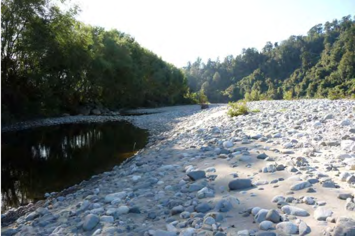
Figure 14 Isolated bank protection works on the left bank of the lower Seddonville reach
