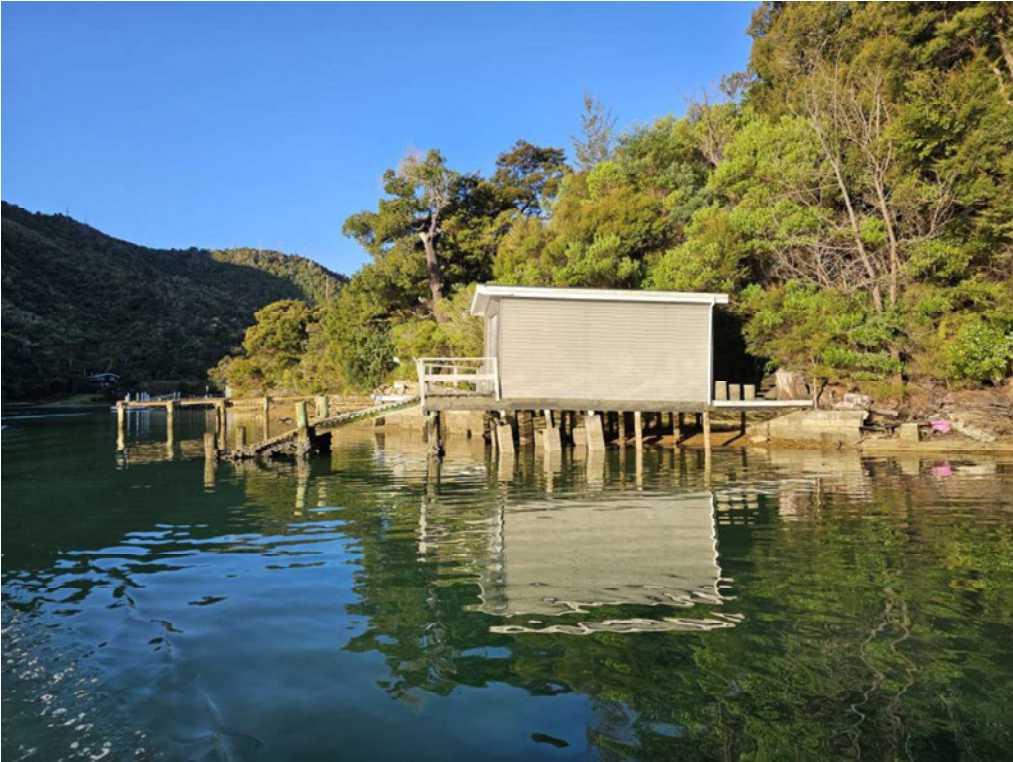
Photo 4: Boatshed and slipway piles knocked forward, looking east
