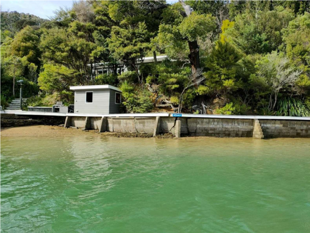
Photo 3: Stairs to foreshore, access deck, small shed and damaged concrete wall.
