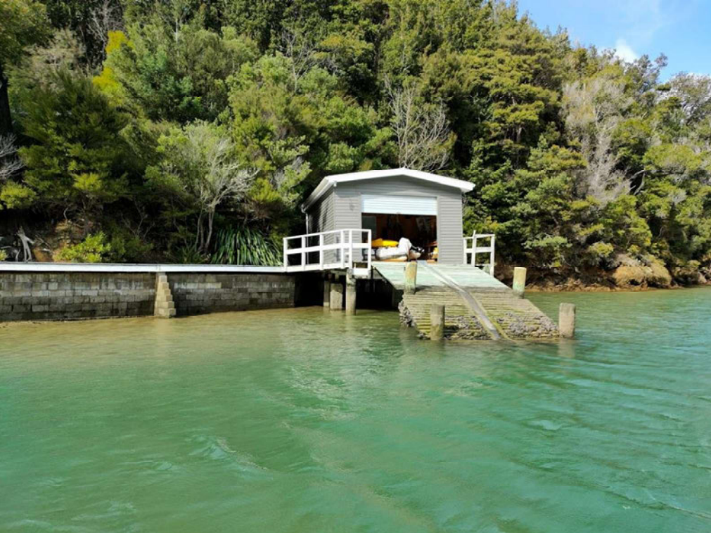
Photo 5: Exiting decking above damaged seawall, boatshed and slipway, looking south
