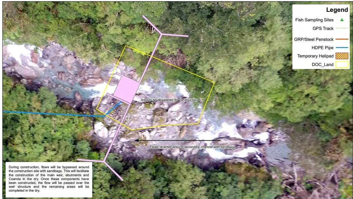
Figure 5: Overview of the works at the proposed intake site on McCulloughs Creek (supplied by No.8 Ltd, 16 August 2017).
