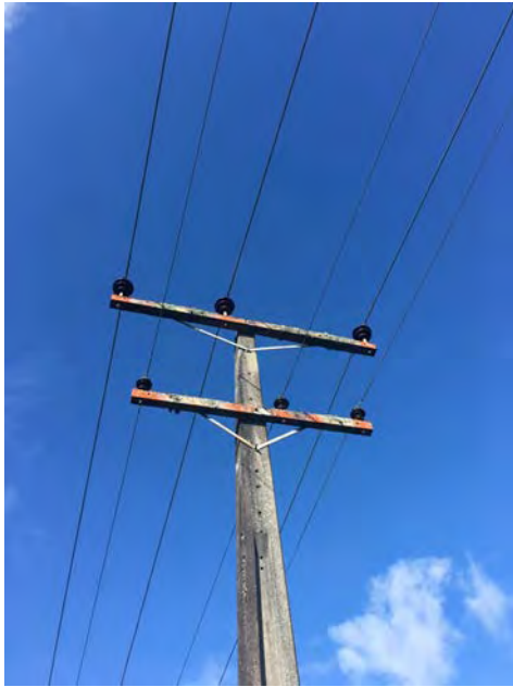
Figure 16 - 11 kV Westpower distribution line
