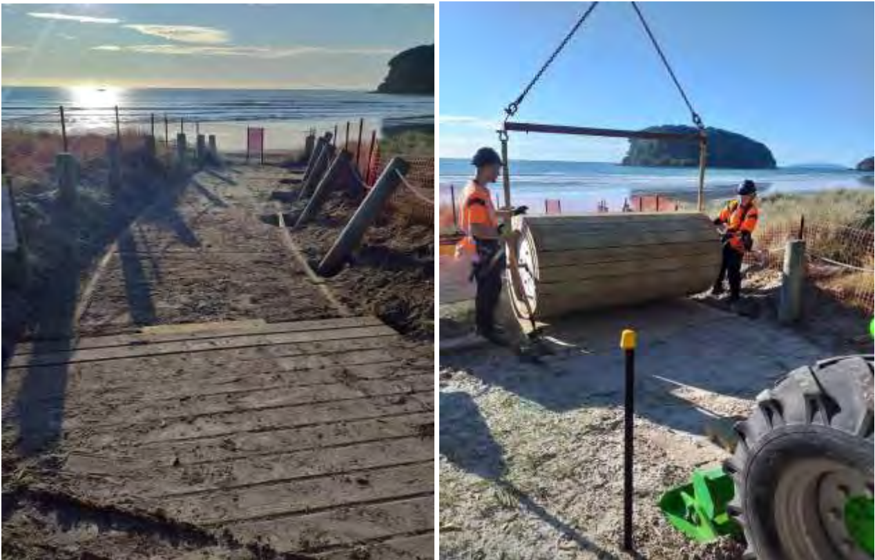
Figures 8 and 9: Showing the recent trial boardwalk installation near the Whangamata surf club.
