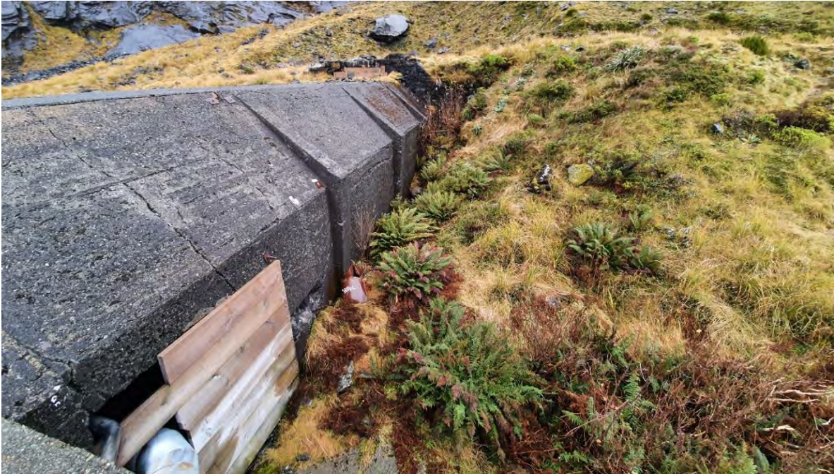
Figure 3-7: Existing avalanche shelter viewed from above existing plant room looking towards stone-faced wingwall at portal entrance
