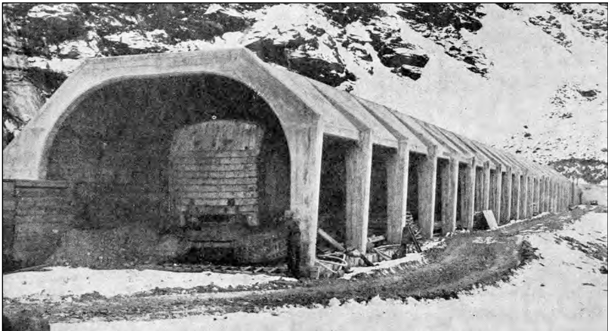
Figure 41. Photograph from July 1940 showing the original extent and design of the eastern avalanche protection. 78
