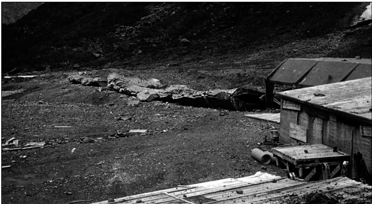
Figure 4. View of collapsed eastern portal avalanche protection, 14 January 1946. 35
