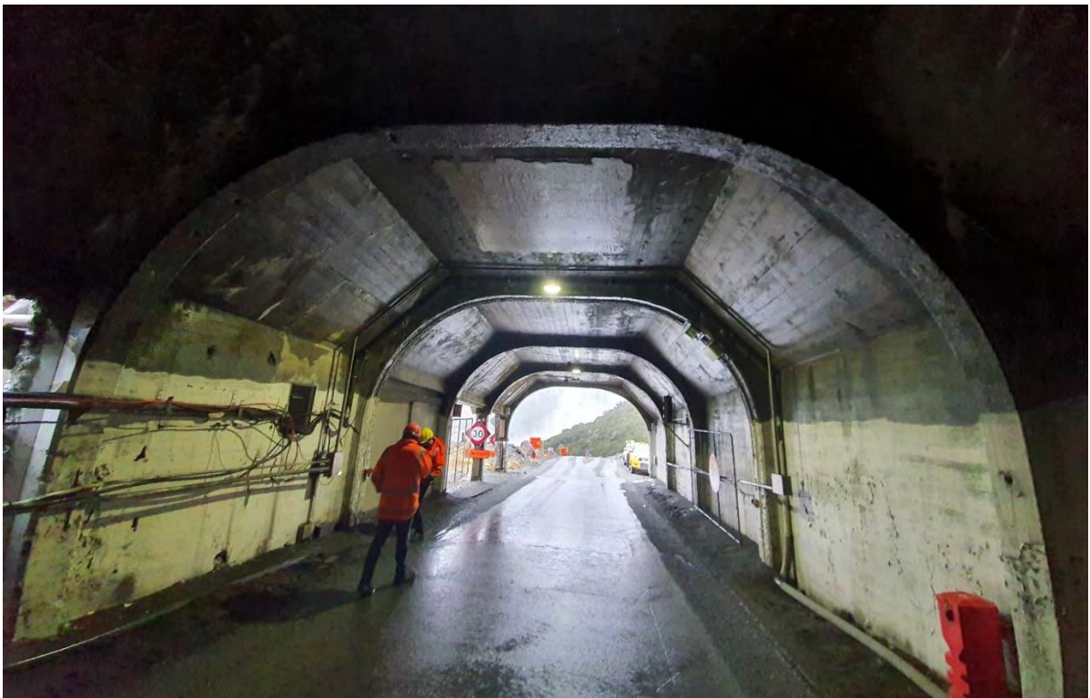
Figure 8-2: Homer Tunnel existing avalanche shelter road entrance as seen from within the shelter.
