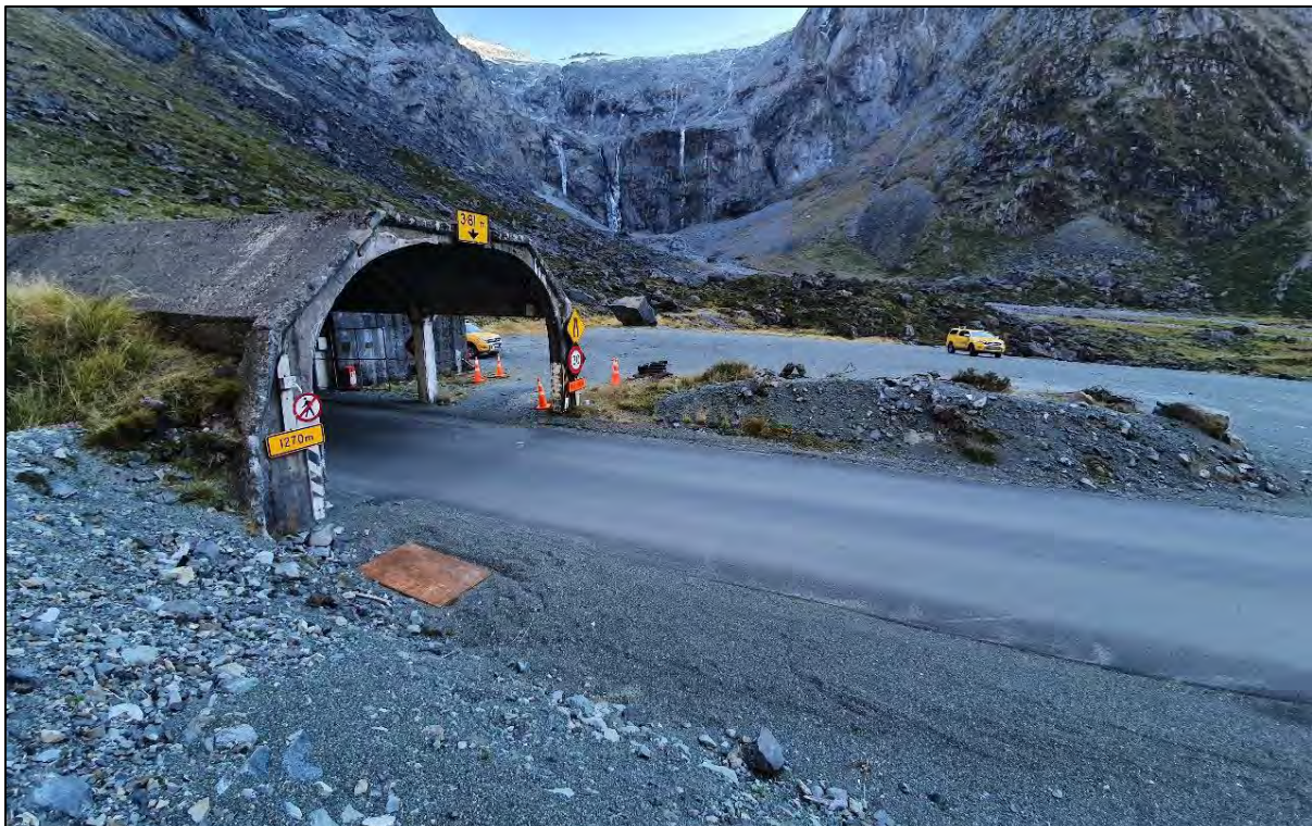
Figure 10. Remaining avalanche shelter and adjacent debris pile.
