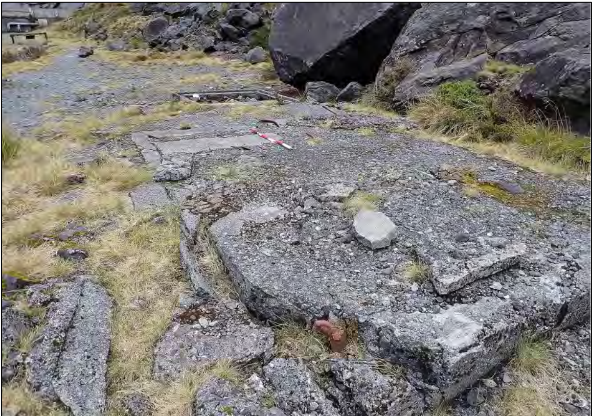
Figure 16. Foundation pads at the workshop site, looking back towards the tunnel portal. The avalanche shelter and plant room are visible at the top left corner. 45
