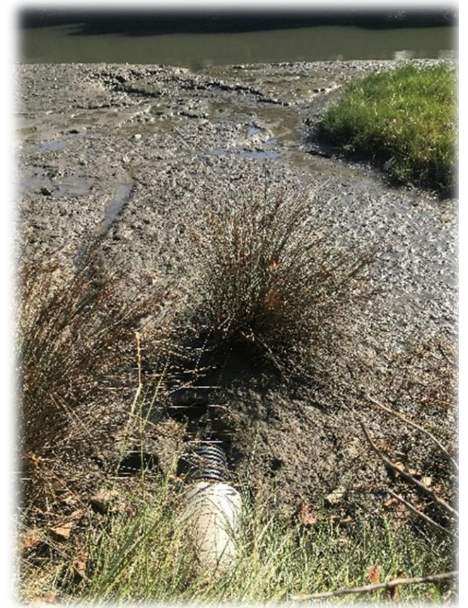
PHOTO 3.21 (i) Stormwater outlet into the river The outlet from roof water - clean.
