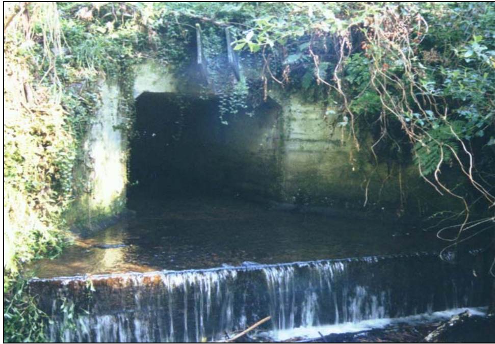
Plate 2. Concrete box culvert. Note the wide cross-section resulting in a thin stream of water over the bottom, and the drop at the end of the concrete pad that is a barrier to swimming species.
