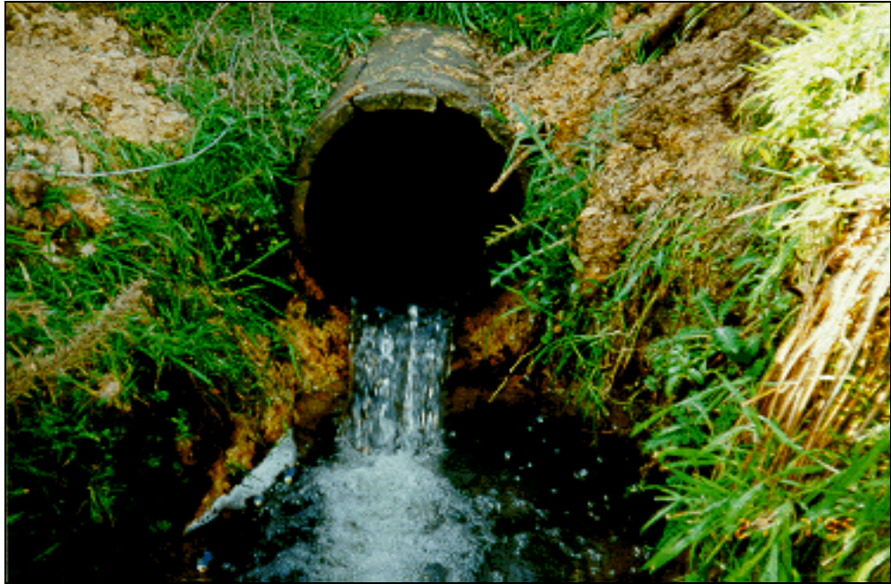
Plate 1. An elevated outlet created either by poor positioning at construction time, erosion from high-energy water exiting the culvert, or erosion from down stream.
