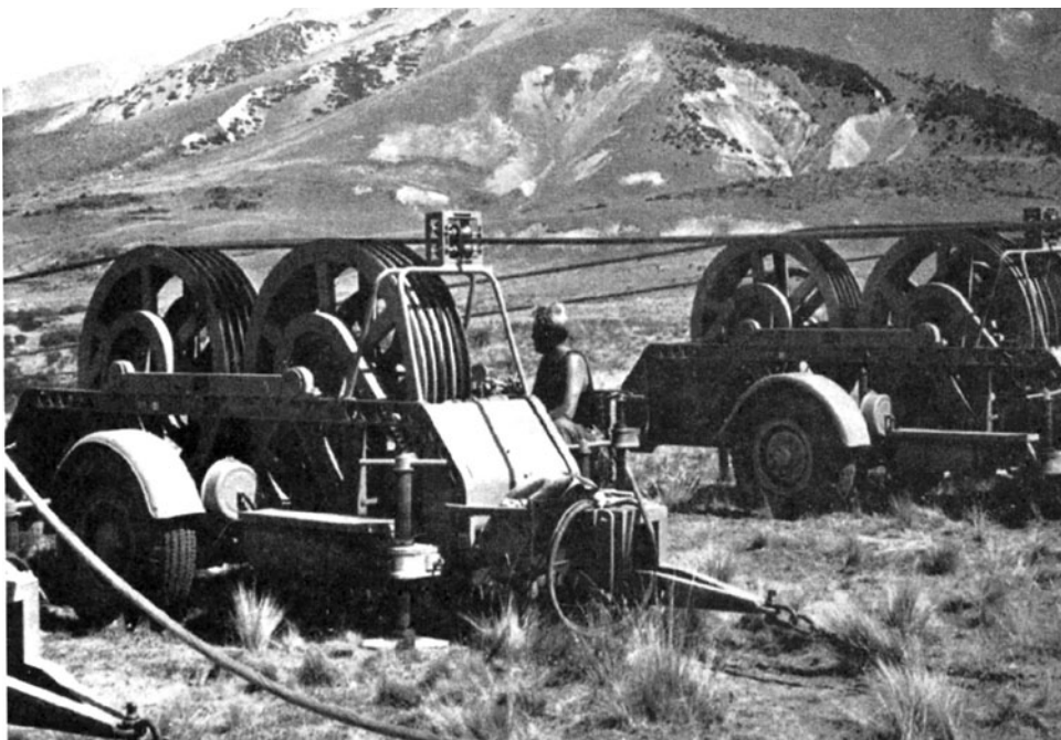
These tensioning winches were used to string the conductors (power lines) between the towers on the 500 kVDC line through Molesworth.
