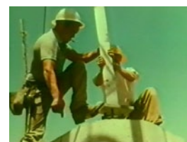
These screen captures from a 1960s N.Z.E.D. film about the construction of the HVDC link show surveying, digging and building tower foundations, tower building and finally the stringing of conductors (lines).
