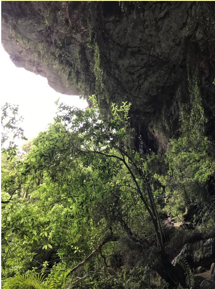
Photograph 3 – Western Limestone Bluff Overhang Section. The proposed track is located at the toe of this bluff and under the overhang.
