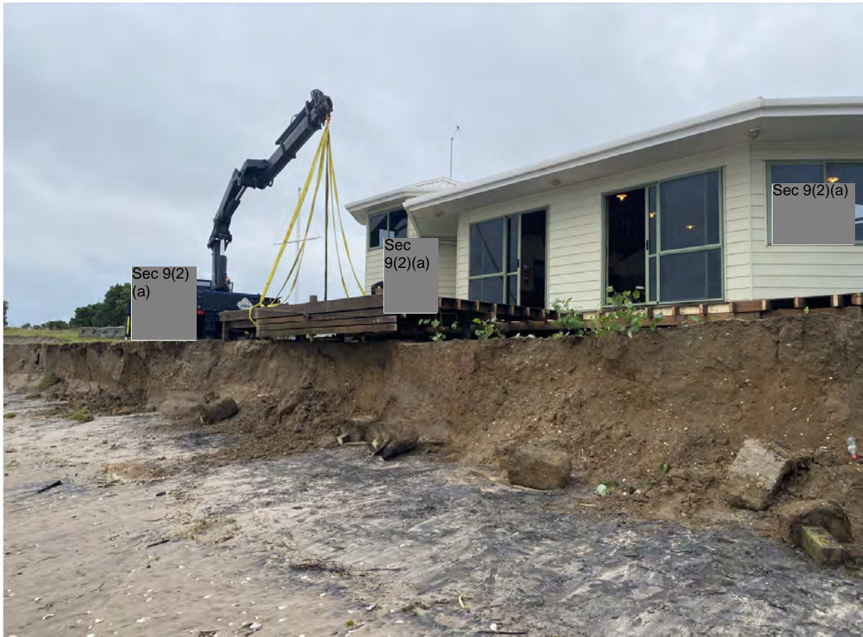
Figure 7 – Erosion and deck removal following Cyclone Hale.
