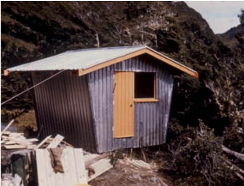
Wisely Hut nearing completion in 1961, with the leftover timbers and iron lying around the site. The hut's distinctive flared walls are easy to see without the later (1976) addition.
