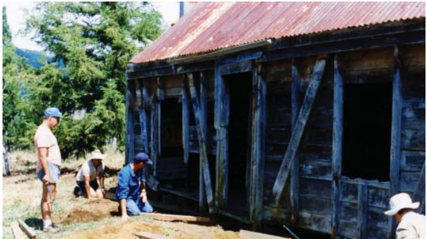
Carpenter Roger Elliott on the left works on the hut while Ongaonga field centre staff Peter Dandy (in the blue overalls) and Peter Abbott watch Dave Rogers at work under the hut.
