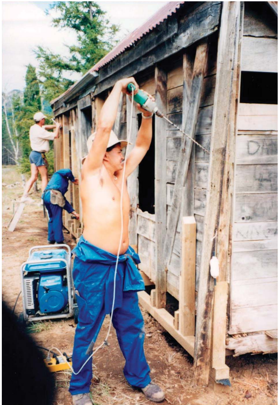
Taranaki conservation officer Dave Rogers drills holes in the original timber of the hut before preservative is pumped in. Behind him is carpenter Roger Elliott who works at the Rimutaka Forest Park for the Department of Conservation, and Peter Dandy, centre, from the department's Ongaonga field centre.
