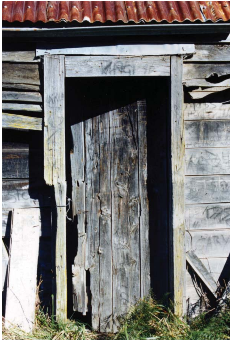
Detail of front door. Replace board on latch edge of door only.
