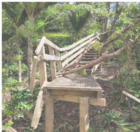
Mt. Manaia Walkway, Northland. Source: DOC damage inspections
