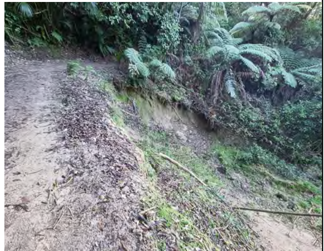
Figure 2. Typical translational slide below the track close to Anapai Bay.
