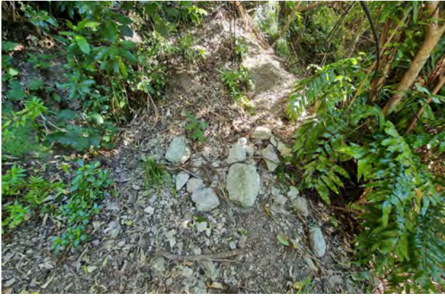
Figure 11. Small scale rockfall on the track at Ratakura Point.
