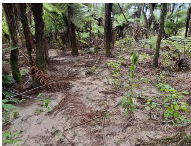
Figure 18. Track inundation damage caused by the debris flow shown in Figure 17 (Bark Bay).
