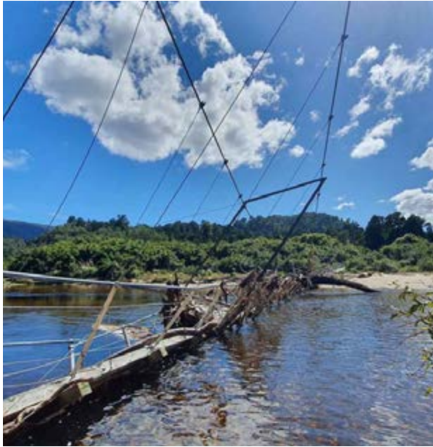
Damage to the Heaphy Bridge. Photo: DOC
