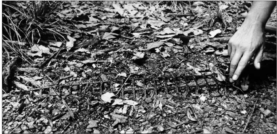
Figure 23. Open-pored moulded geogrid provides a base for well-bedded angular gravel protecting a midden on this track in the Ohope Scenic Reserve, Whakatane.
