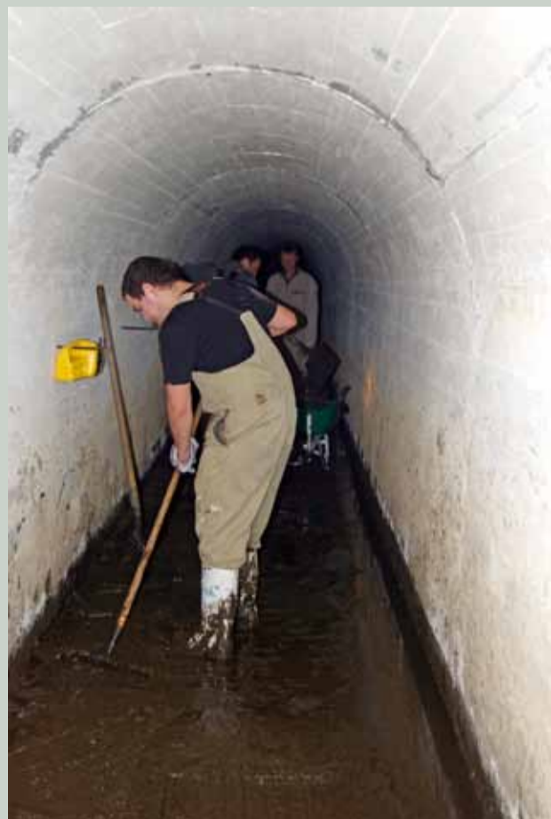
Washing mud and debris out of the plotting room tunnel network, Motutapu Island. Photo: Jonathan Canning
