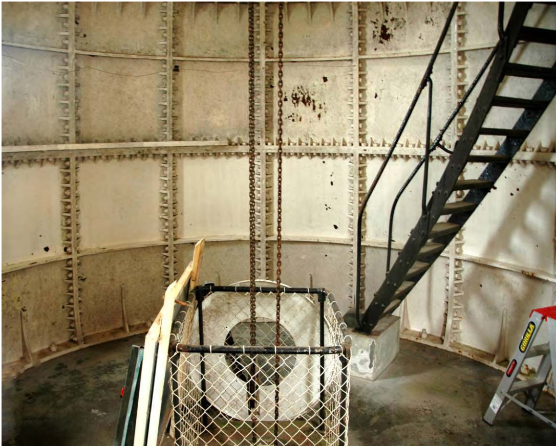
Figure 195 – The bottom floor of the lighthouse during cleaning. Here the flaking paint has been scraped, the floor swept and one row of panels has been scrubbed, 2008.
