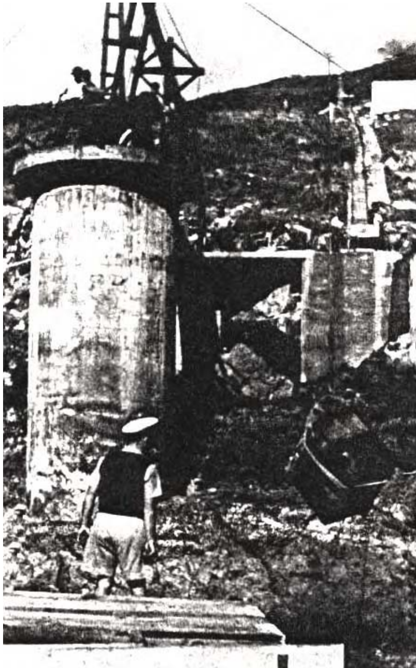
Figure 36 – The view of the gantry from the stores boat during World War 2.
