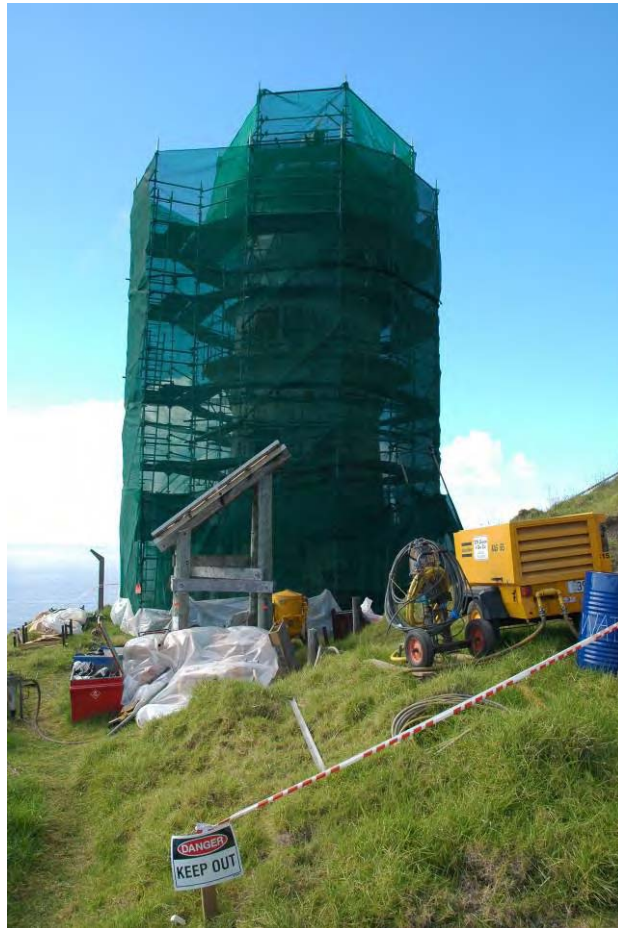
Figure 34 – The worksite during the paint work with the lighthouse covered in scaffolding.
