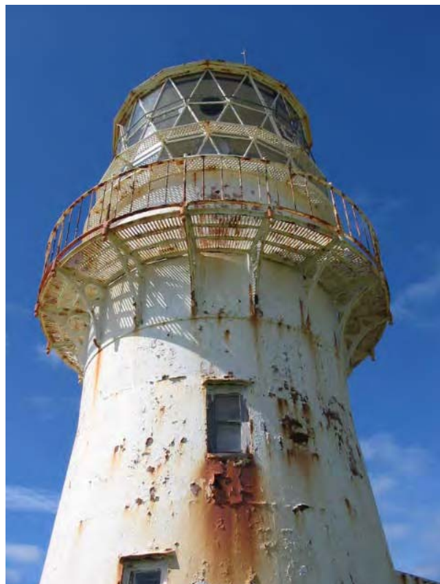
Figure 33 – The lighthouse before being painted in 2007.
