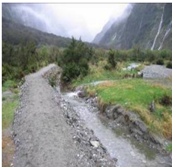
Figure 41 -This raised formation on the Milford Track works well having raised the walking surface above the surrounding ground surface. Raising the track means the pressure now applied to the natural ground surface is very low; this prevents failure of the natural ground surface
