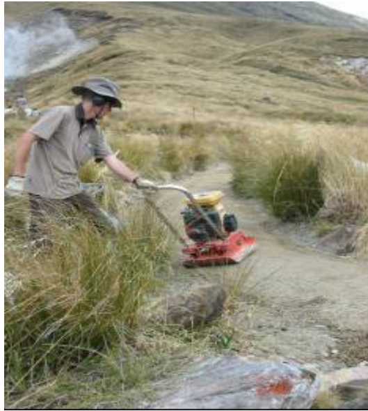
Figure 11 - Use of a vibrating plate compactor helps to harden the track surface and reduce erosion and displacement of material
