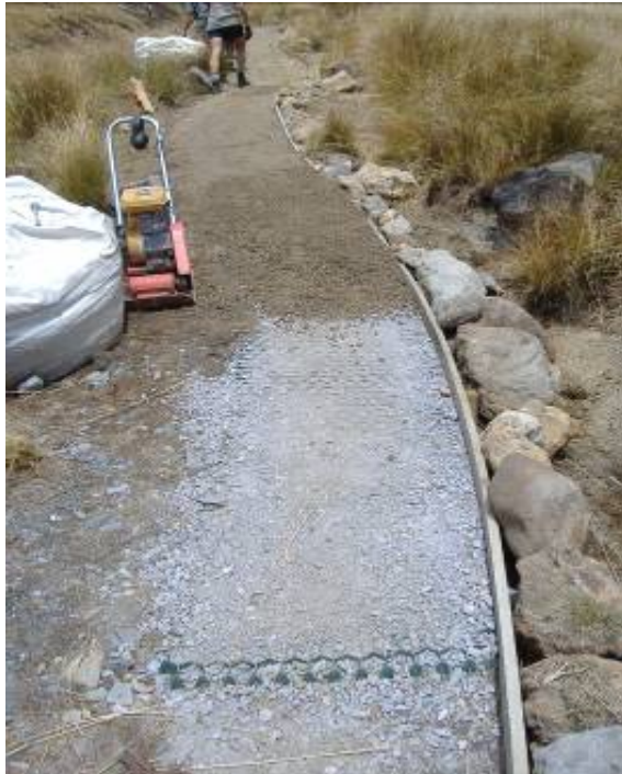
Figure 58 – With the geocells filled the walking surface can be applied and compacted
