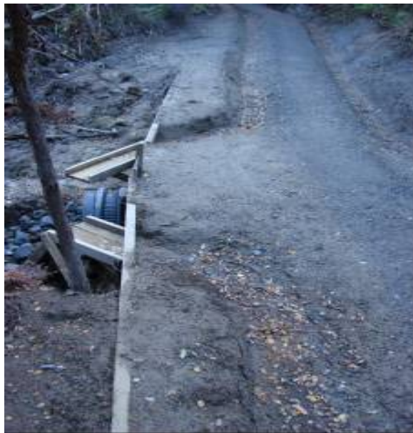
Figure 39 - This track has large side drains on either side of the walking track. The drop at the end of these timber chutes and culvert can cause water to erode the soil. Some form of soil erosion protect would be required
