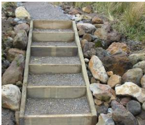
Figure 79 – Completed set of stringer box steps. These will require very little maintenance for a considerable period of time
