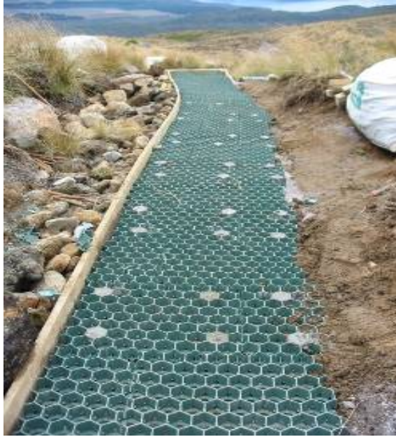
Figure 57 – To hold the cells in place a 12 mm reinforcing rod is driven into the soil. The individual cells containing the rods are then filled with a hardener to secure the geocells in place.
