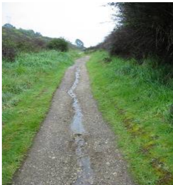
Figure 101 - Several factors are contributing to the scouring evident on this track. A seepage spring has surfaced in the middle of the track, the track is poorly shaped and erodible track surface material has been used
