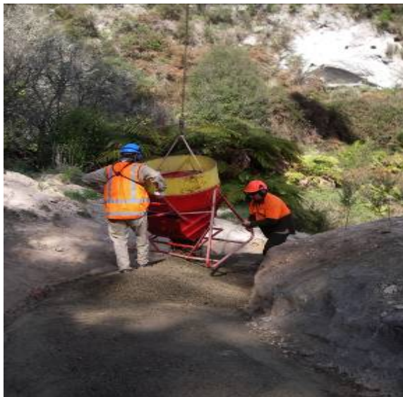
Figure 69 -Use of a hopper is a very efficient method of spreading stone aggregate. By calculating the volume of the hopper you can determine how far one load should be spread to achieve a finished compacted surface 50mm thick
