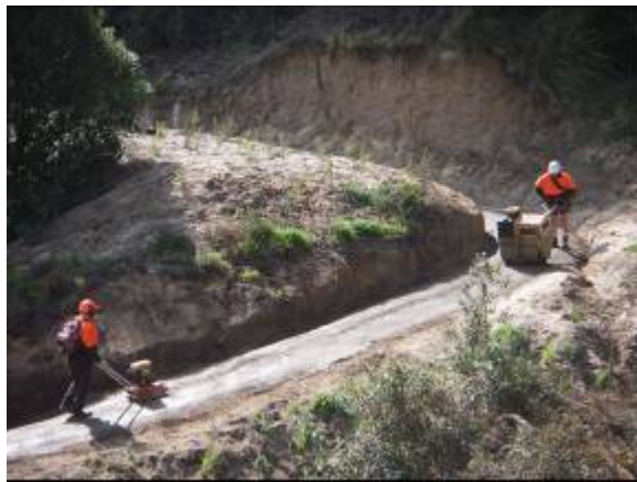
Figure 52 - Working in tandem is the vibrating plate compactor, bottom left, followed by the static roller. Note the track has been compacted from the outside edges to the centre
