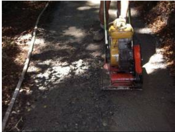
Figure 51 – Good compaction technique. Compaction commenced on the outside edge and each pass of the vibrating plate compactor is overlapping the previous pass
