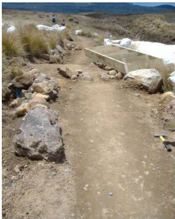
Figure 73 - During the track survey information on step construction is obtained. This allows prefabrication of stringer steps before being transported to the site
