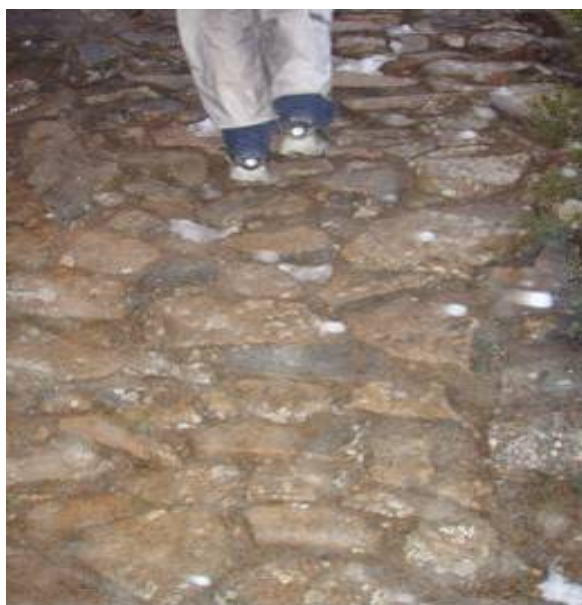
Figure 42 - Stone pitching, while very labour intensive to construct, will last an exceedingly long time
