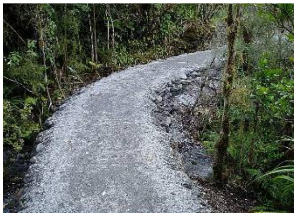
Figure 43- This raised track has a pavement consisting of a base of moraine boulders sub- base of AP65mm and surface of AP20mm
