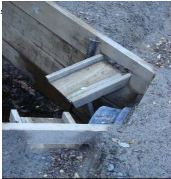
Figure 40 - This outlet is far too small for the size of the side drain. Furthermore, beech forest drops an excessive amount of leaf litter (accumulation of material is evident in the side drain) and this will further block the outlet
