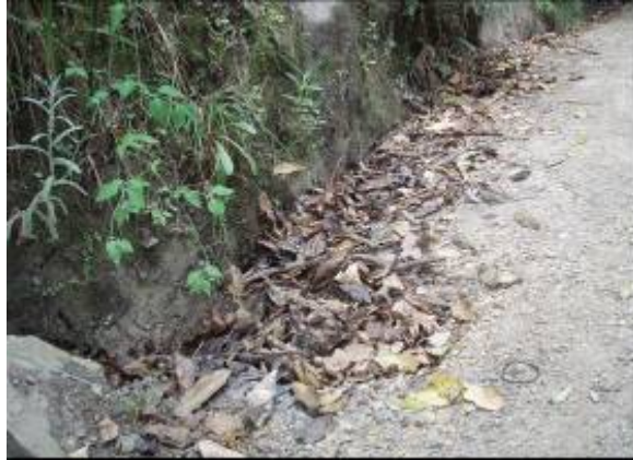
Figure 38 - Side drains can easily collect a large amount of leaf litter in a short period of time, compromising their effectiveness. Side drains need to be maintained regularly
