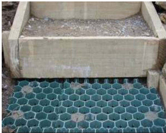
Figure 78 - Geocells have been placed under the first riser to prevent track erosion. In extreme wet weather water will cascade over the riser lip and down onto the track surface
