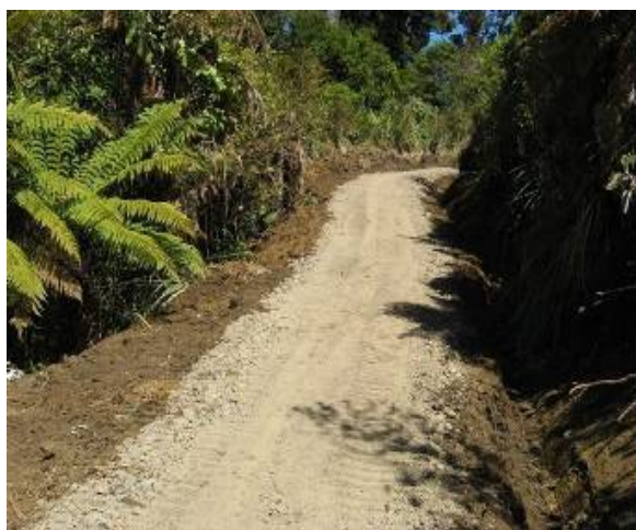
Figure 48a - Larger stones have been pushed to the side of the track when compacted as the material lacks angular stone structure (section 15.5.2)
