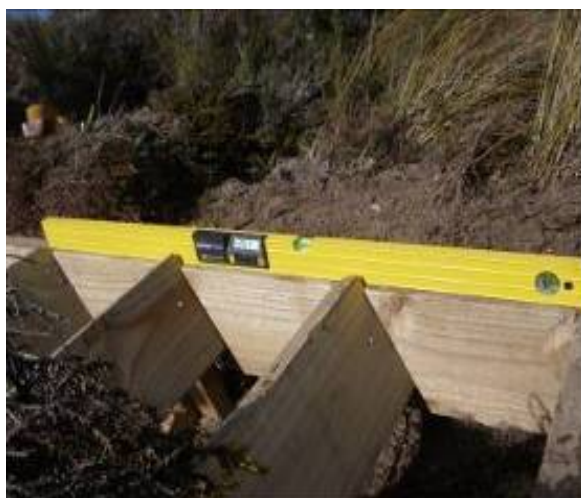
Figure 74 - Use a level with a digital display to get the steps at the correct gradient
