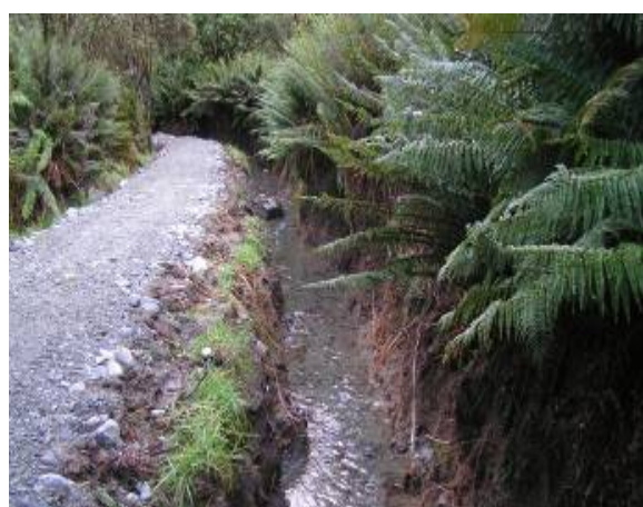
Figure 99 – In extreme rain events this side drain has been almost full
