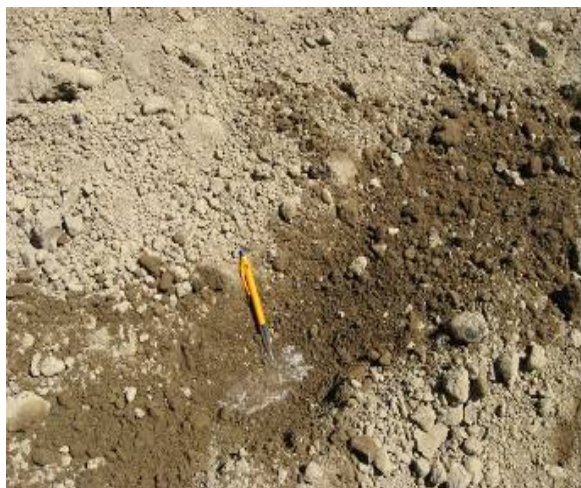
Figure 47 - When transported to site and compacted, poorly graded material is easily displaced
