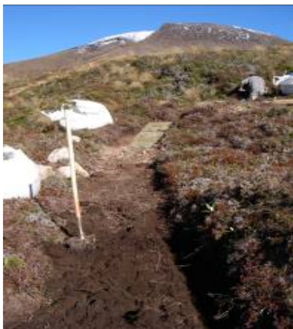
Figure 54 – Removal of organic material is required. If a track was built on top of the vegetation, movement of the track surface would take place as this decomposed
