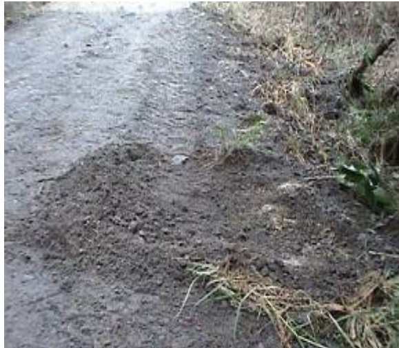
Figure 100 - This poorly graded material has been transported to the side of the track through displacement and erosion.
