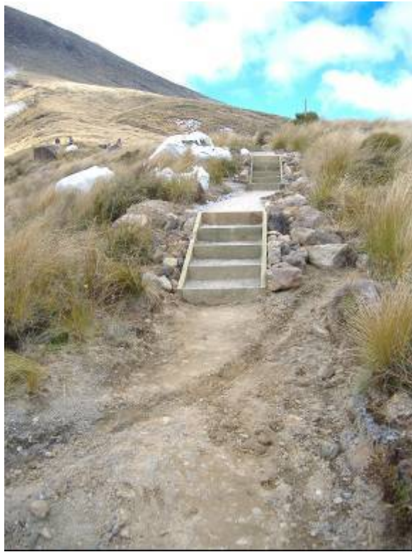
Figure 77 - The side drains have been lined with rocks to slow down the water in this very erosion prone volcanic ash.
