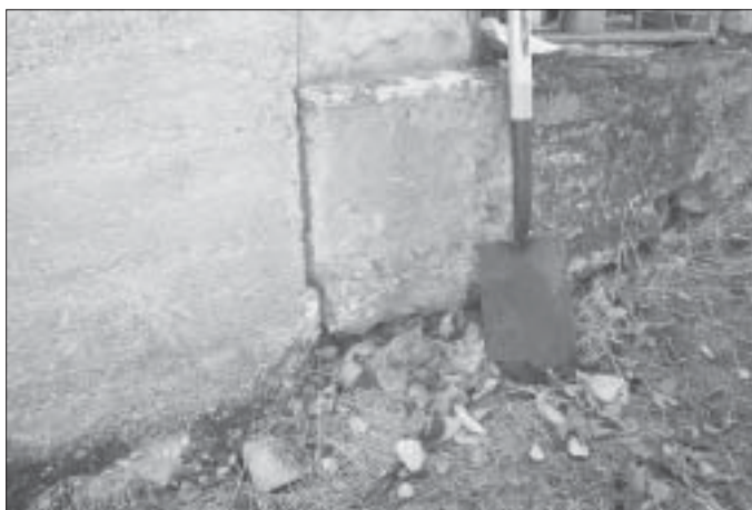
Figure 25. Rear right-hand storeroom. Failure of 'recent' concrete foundations cast at ground surface.
