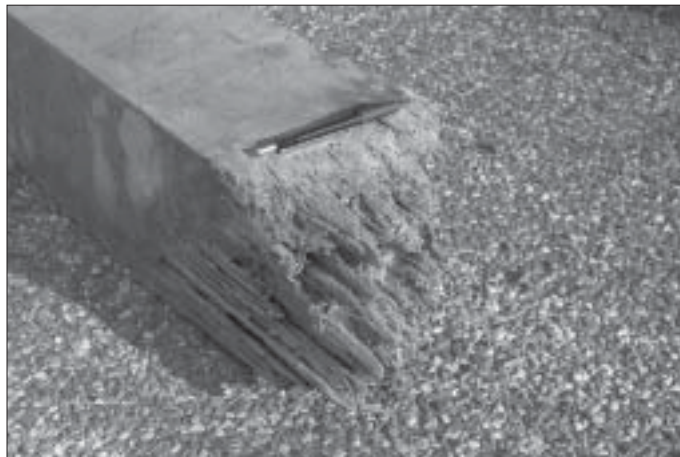
Figure 17. Timber pile shown in Fig. 16 above. Note severe rot at contact with ground.
