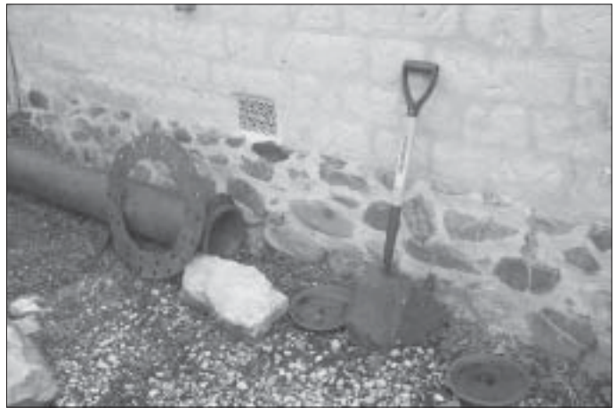
Figure 32. 'Modern' repointing (and possible rebuild) of cobble foundation midway along right-hand side wall.
