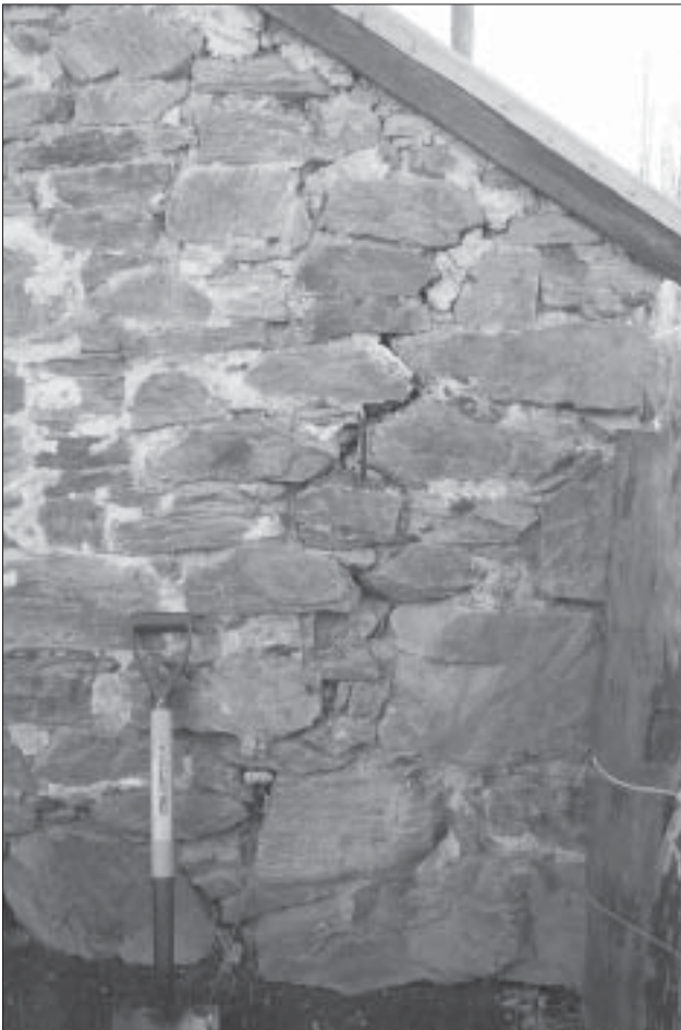
Figure 21. Severe cracking in left-hand wall.
