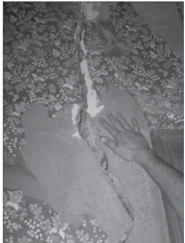
Figure 34. View of re-plastered crack shown in Fig. 33 from inside SWC office.
