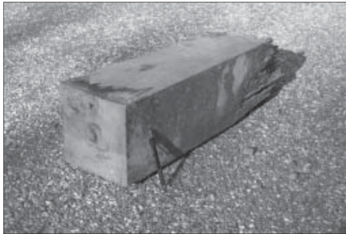
Figure 16. Example of timber pile replaced during 2000 levelling works.
