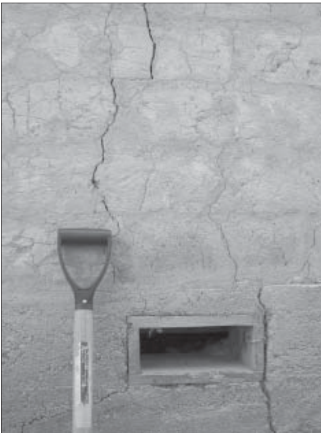
Figure 27. Rear right-hand corner of hall. Note severe cracking of concrete underpinning.
