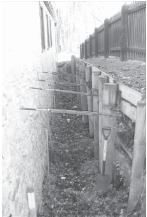
Figure 24. Tie-rod system along left-hand side wall. Before the retaining wall was installed, the ground had built-up against the foundation wall, exerting earth pressure for c. 100 years.
