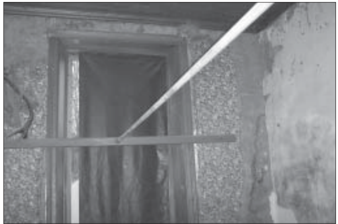
Figure 30. Tie-rod system inside the Scandinavian Water-race Company (SWC) office—view of front wall.
