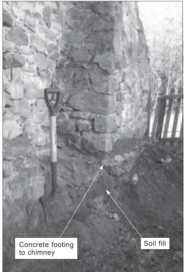
Figure 22. Recent soil removal on left-hand (uphill) side has relieved earth pressure on the wall, but undermined the footing to the chimney.
