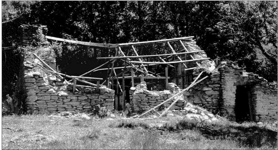
Figure 2. Front (north) elevation of Needham's cottage prior to restoration in the late 1970s. 2 Photo: L&S records from DOC files.
