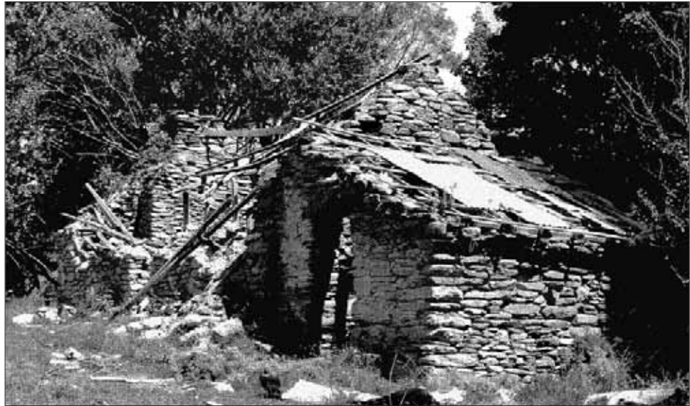
Figure 3. Needham's cottage from the west, prior to restoration in the late 1970s. 2 Photo: L&S records from DOC files.
