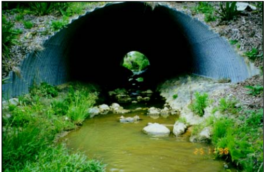
Plate 11. Fish-friendly culvert illustrating the “stream slope design option
