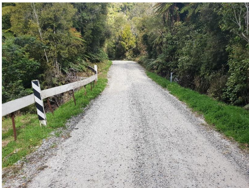
Figure 33. showing a pinch point where a replacement sight rail will need to be installed and rock armoring may be required. The vegetation has a moderately high degree of naturalness but will likely be little affected because of an adequate amount of room to expand the road width without intruding far beyond the existing low stature vegetation/existing drainage channel.
