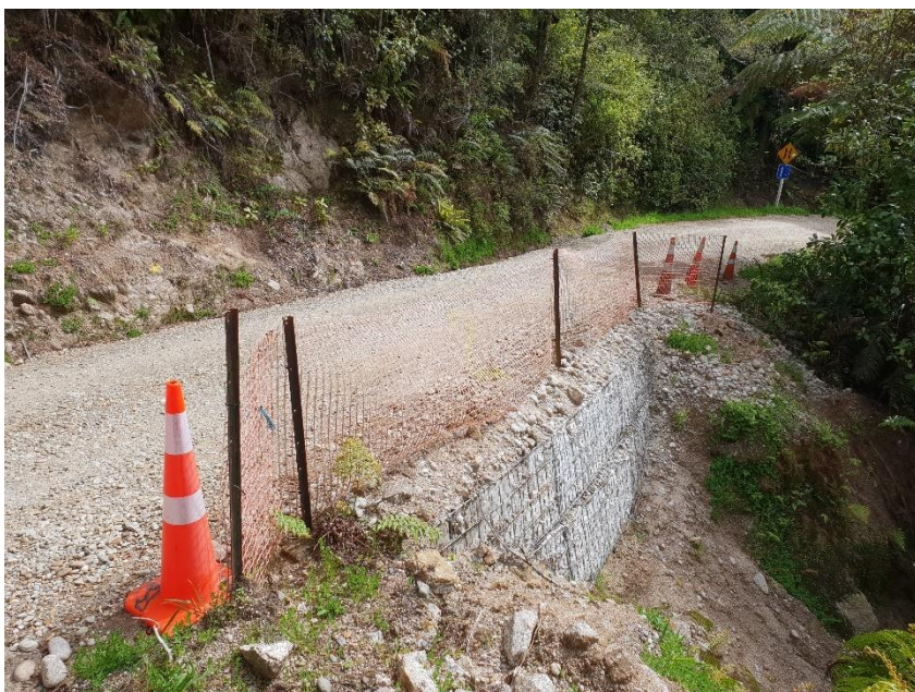
Figure 41. A typical site where rock armouring/gabion baskets might allow better utilisation of modified habitat and reduce the amount of indigenous vegetation clearance on the opposite side of the road.
