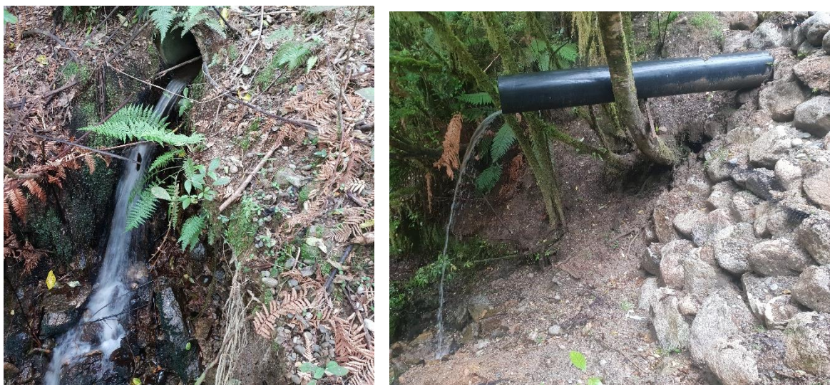
Figure 34. Culvert 035 is perched by about 1.5m and has a very high flow, and yet surprisingly was the smallest catchment in which banded kokopu were found (as well as koura), about 50m upstream of the road within a forested catchment.
