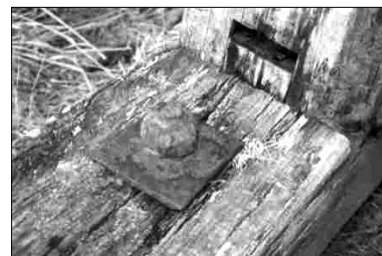
Figure 6. A steel washer on the 'Come-in-Time' stamper battery in the Bendigo Reserve Area, Central Otago.
