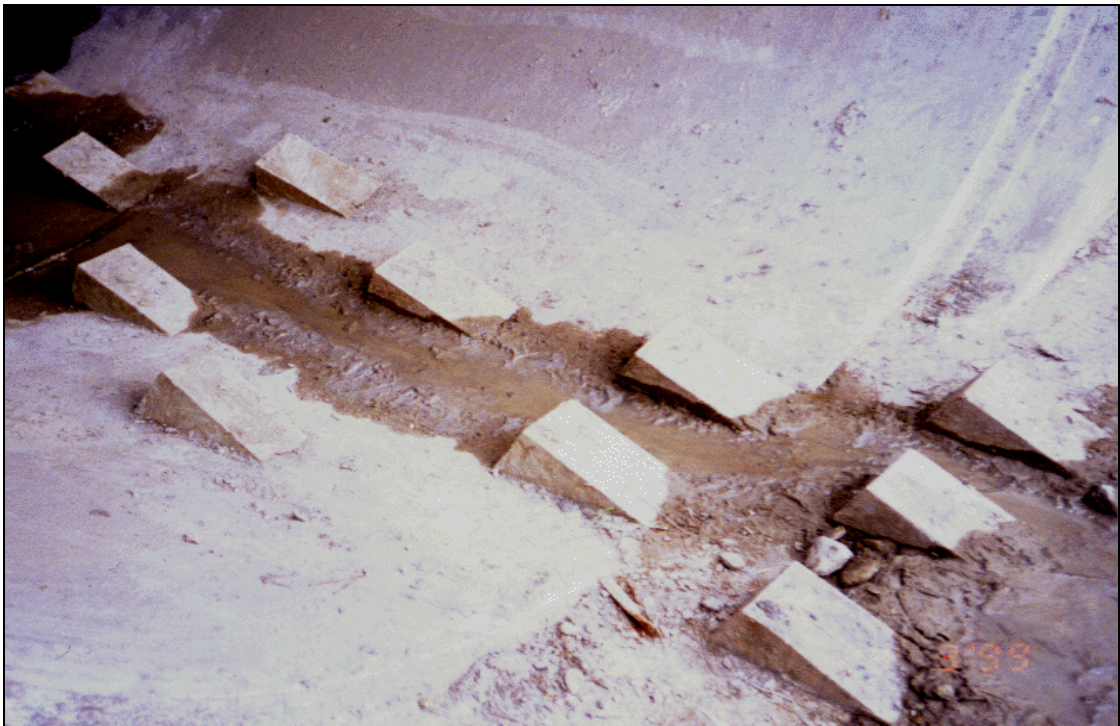
Plate 8. Tanalised pine spoilers installed on the invert of a new concrete culvert. Once water is restored to this culvert it will flow from right to left.
