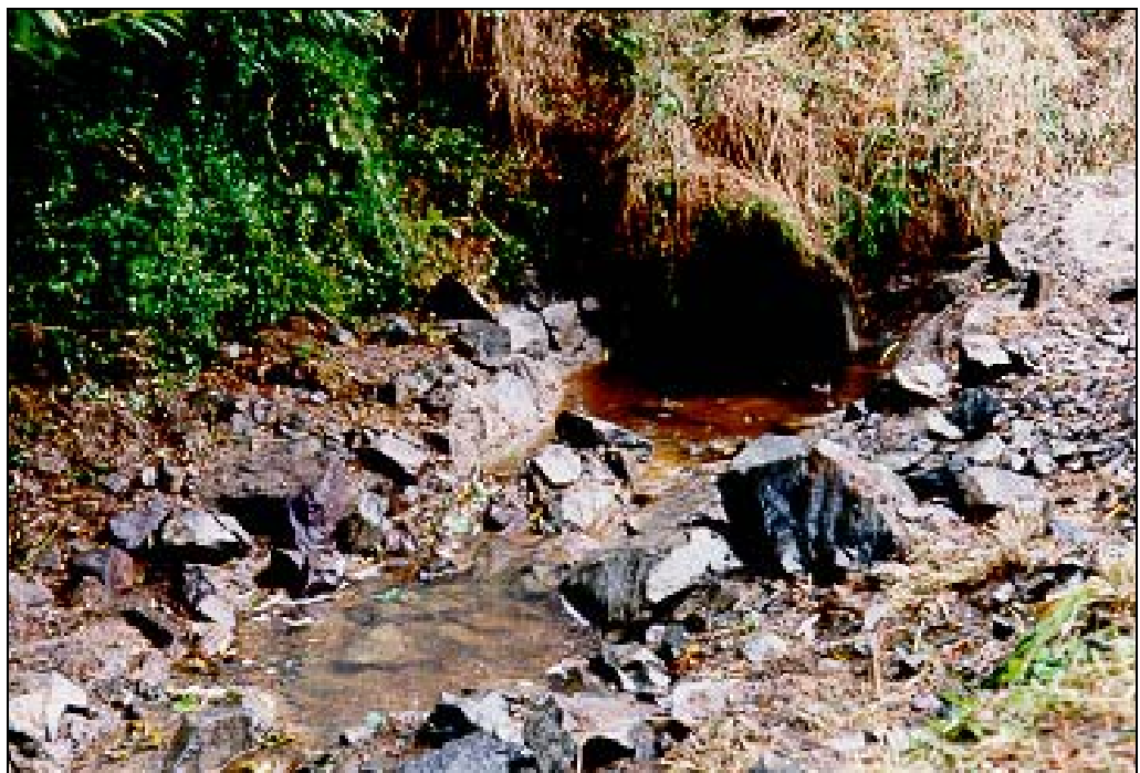
Plate 10. Outlet pools created by a series of small rock weirs. Such pool and weir structures provide resting areas, eliminate elevated outlets through backwatering, and decrease barrel velocities at low flows.
